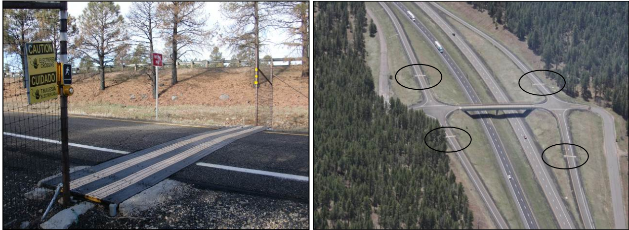
Figure 10. Electrified Cattle Guards Installed at Schnebly Hill Road TI (Left) and at Fox Ranch Road TI (Right; Guards Circled)
