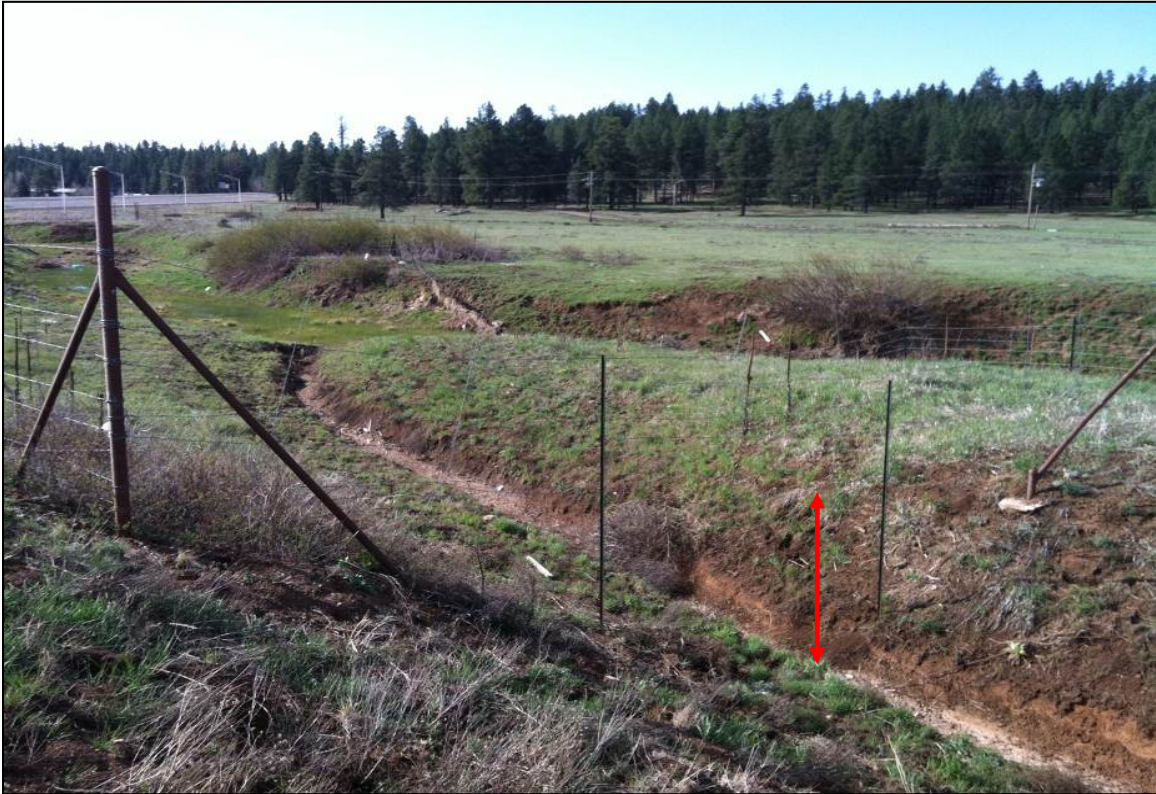
Figure 24. Example of Wash-out (Red Arrow) Near Site of an Elk-Vehicle Collision in 2014
