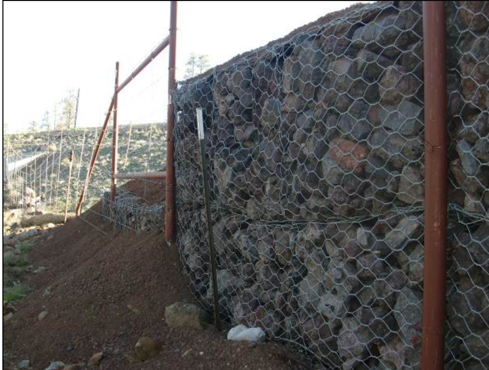
Figure 26. Photograph of Erosion of Interstate 17 Jump-outs
