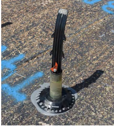
Figure A-7. Sample 4T Failure at 56 Impacts.
