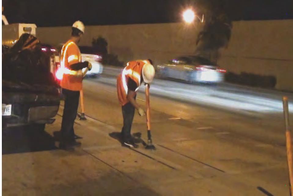
Figure 3. Sheeting Failure and Post Failure Replacement.
