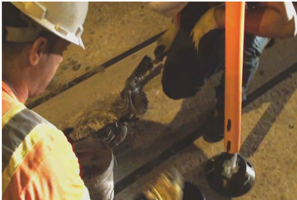
Figure 5. Epoxy Failure and Pavement Failure Replacement.
