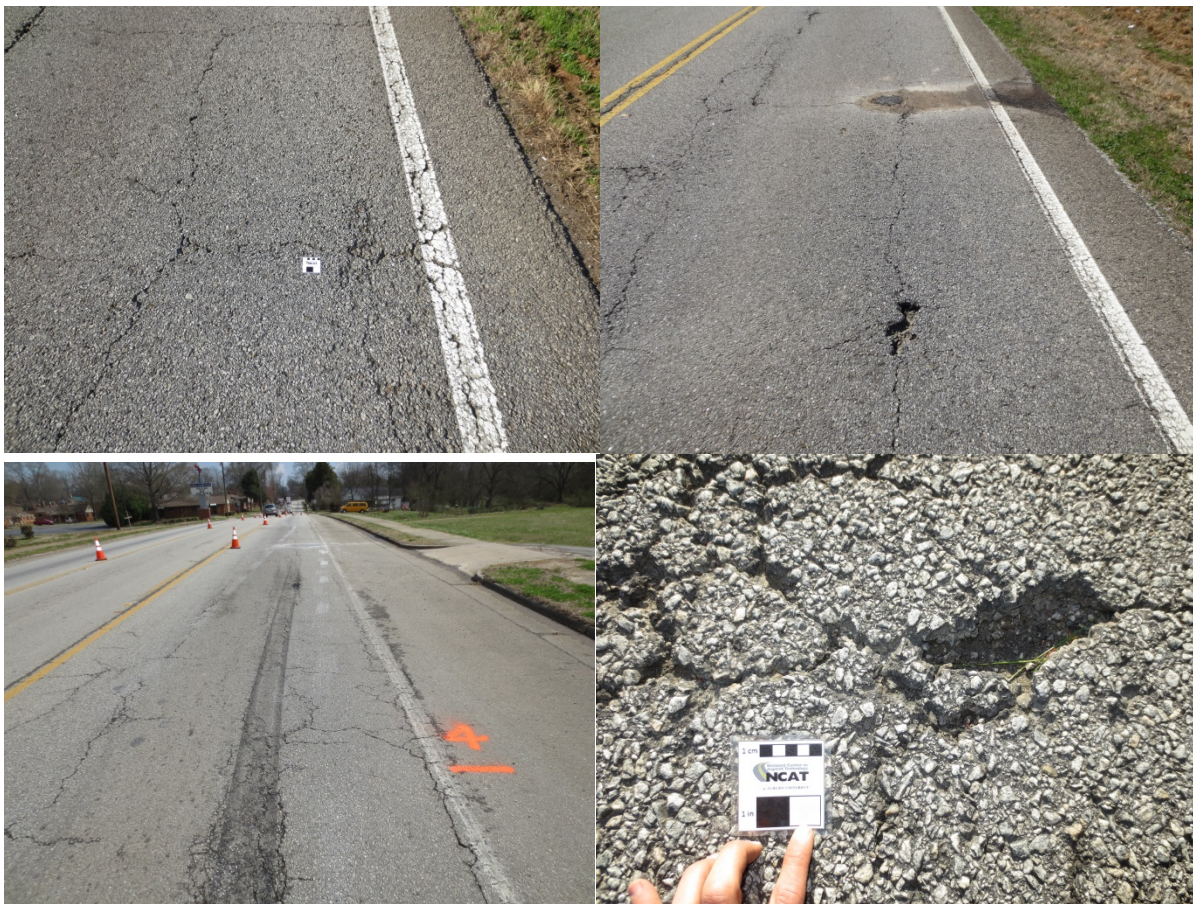
Figure 5—Examples of Distressed Pavement with Higher Amounts of Cracking
