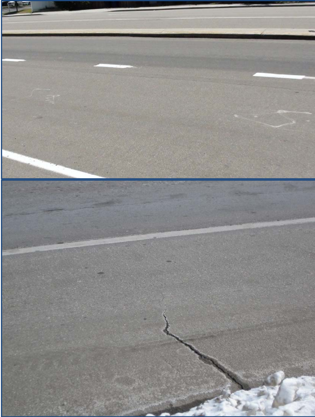
Figure 5-5 SR 111 on June 13, 2012, no visible thermal distress (Top) and January 23, 2013, showing a thermal crack (Bottom)
