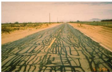
(a) Overtreated Cracks
