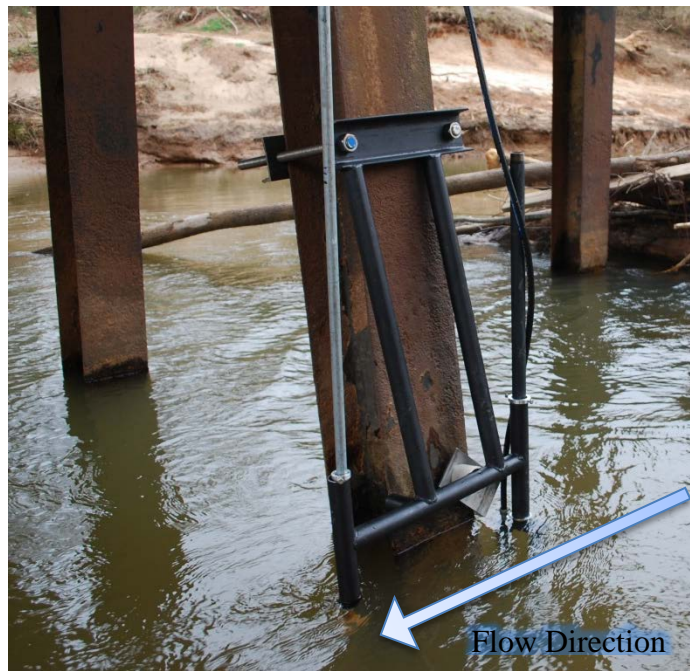
Figure 6.8: Installed TDR (on the right) and sonar (on the left) at Field Site 2.
