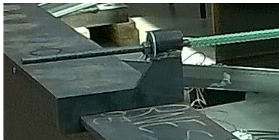
Figure D.2 Transverse tie connected to Dayton Superior C137 tie bar beam clip pre-stress hanger.
