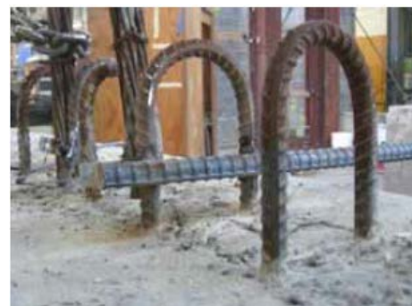
(b) Transverse tie bar (connected from exterior girder to first interior girder), welded end (Yang 2009)
