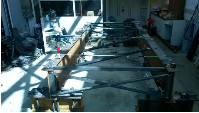
Figure D.47 Cross frame not at midspan + 2 diagonal pipes + 4 transverse ties (1-CF@ 3.5 ft. from midspan + 2-DP + 4-TT).
