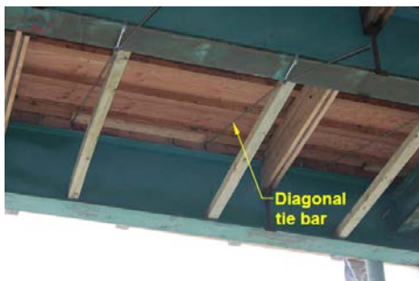
(a) Diagonal tie bar (connected from exterior girder to first interior girder)
