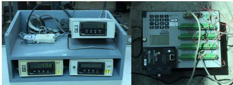
Figure 5.3 Load reading device (left) and data logger (right).
