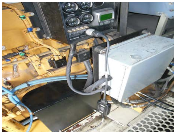
(a) Caterpillar “Electronic Technician” Communication Adapter Connected to the Head End Power Engine
