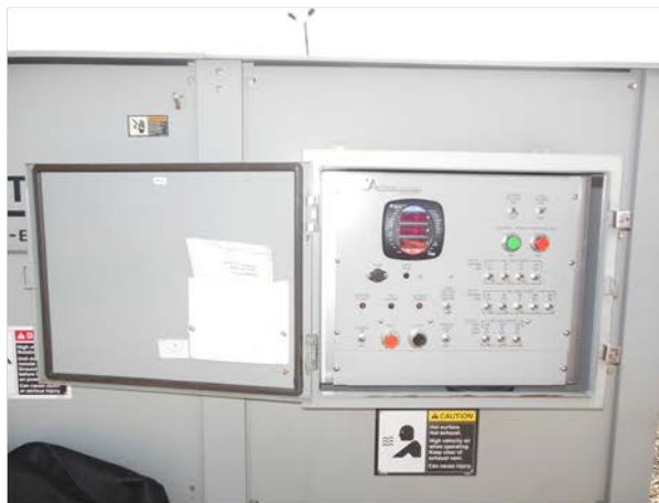
(c) Load Box Digital Control Panel
