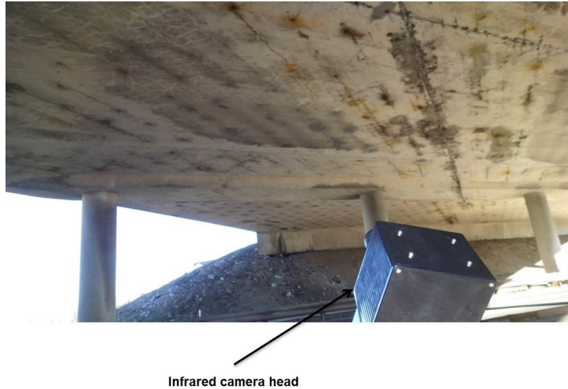
Figure 48. Photograph showing the camera head and the area of the bridge soffit imaged during the test.
