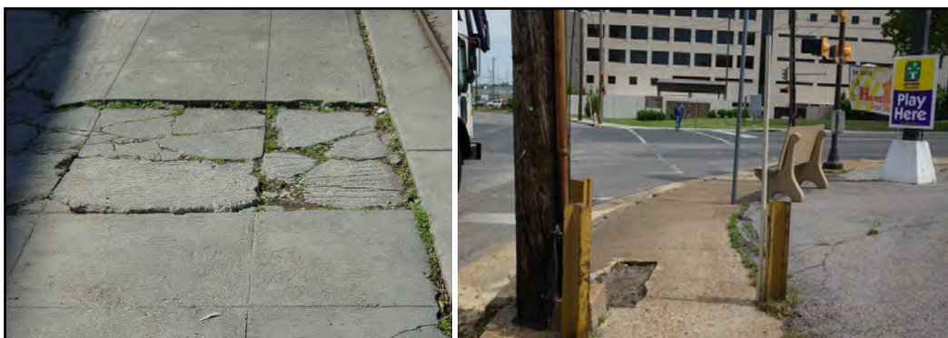
Figure 19. (Left) Uneven, Cracked Sidewalk Surface; (Right) Obstacles Limiting Sidewalk Width and Broken Surface
