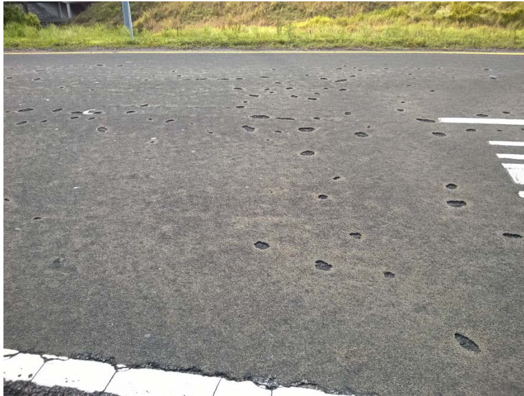
Figure 2.10 – Widespread localized failures due to poor binder mixing (US 90 – I-75 NB)
