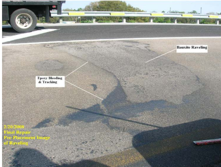
Figure 2.12 – Result of incorrect proportioning: aggregate loss, epoxy bleeding, and epoxy tracking (Polk Co. Parkway to I-4)
