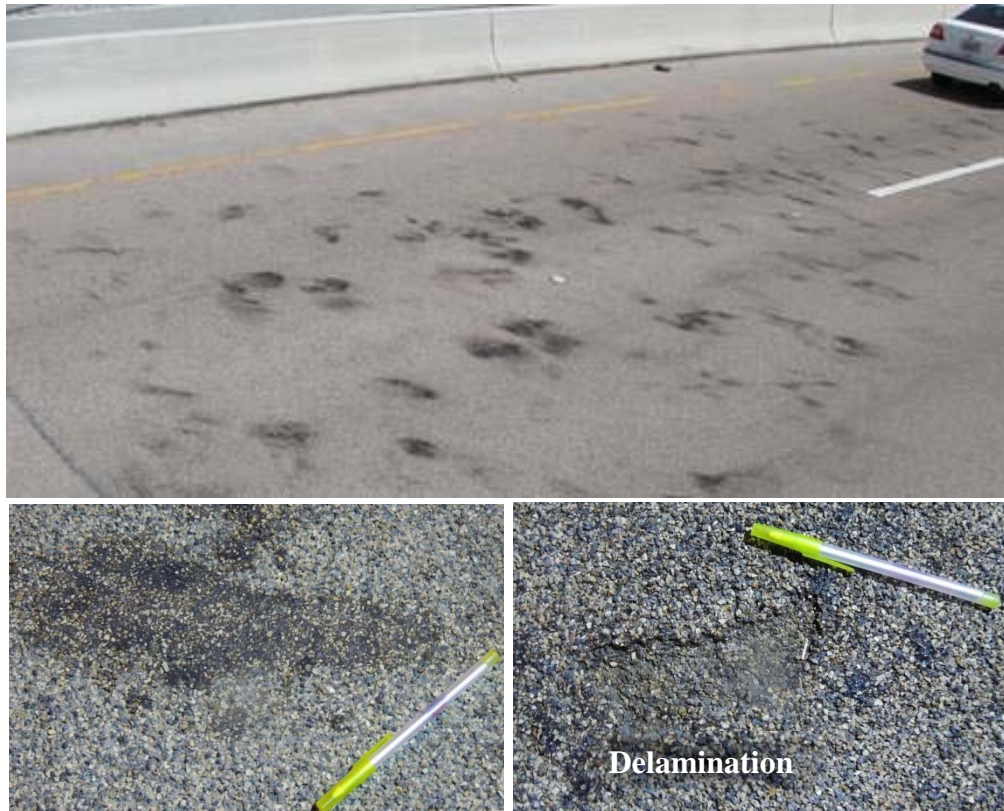
Figure C.16 – Splotchy areas on southbound exit ramp.
