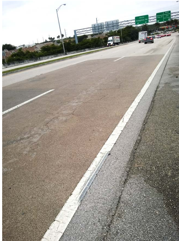
Figure C.23 – Random cracking of HFST after the curve and over HMA.
