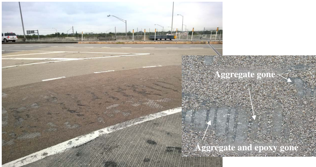
Figure C.22 – Wearing away of HFST around the curve over concrete.
