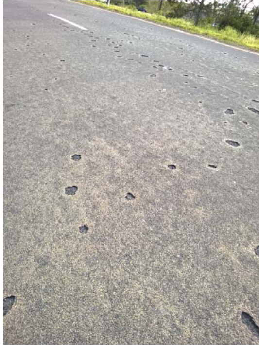
Figure C.6 – Uncured binder failure and potholing.
