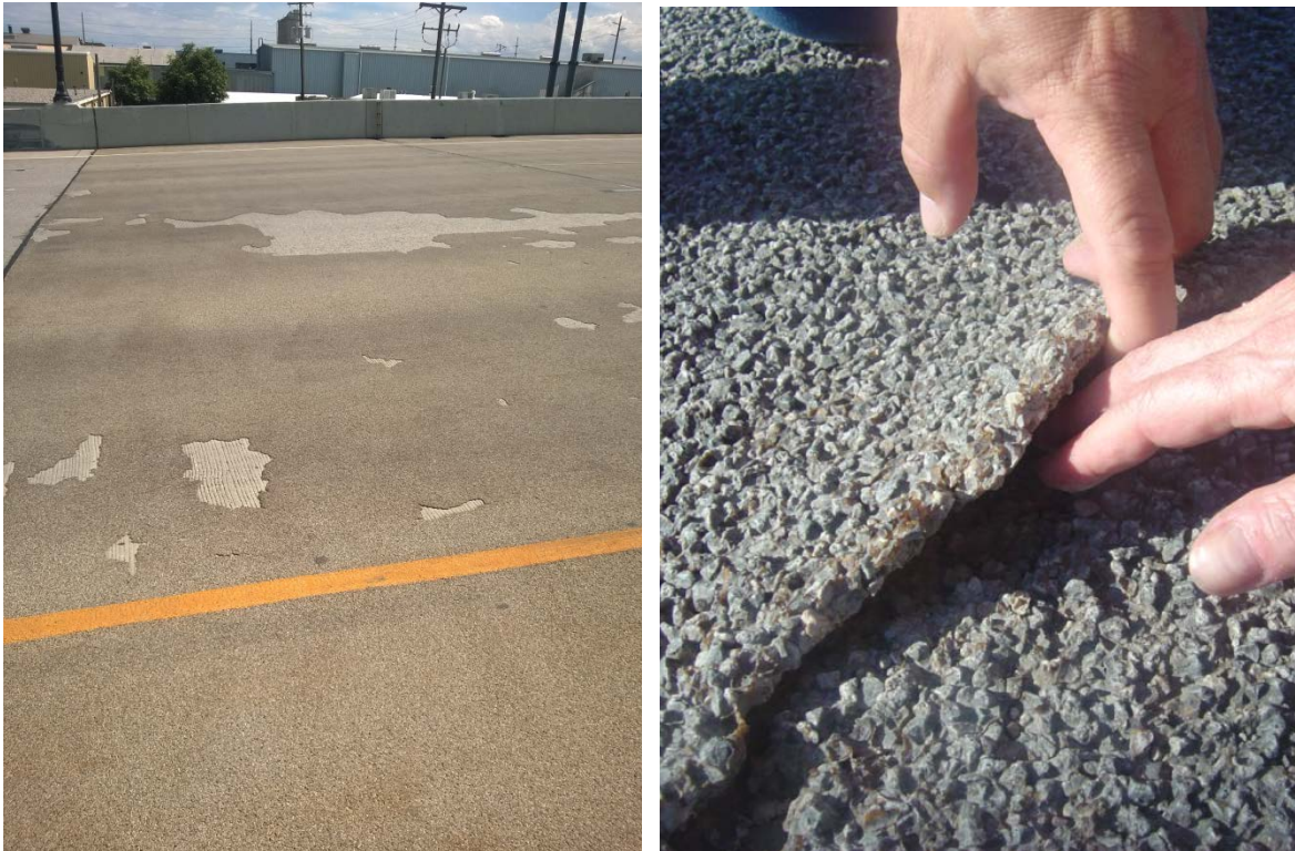
Figure 2.9 – Delamination: Bridge deck and a double layer HFST
