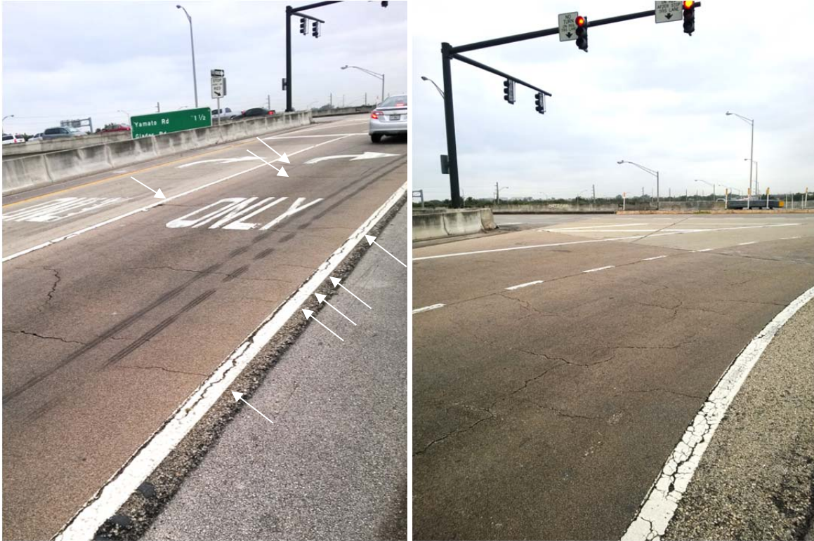
Figure C.21 – Distress near stop bar over OGFC: a) transverse and b) random cracking.
