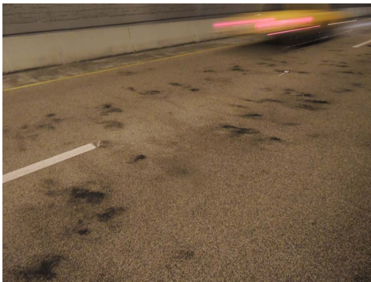
Figure 2.11 – Soft blotchy areas shortly after construction (I-95 ramp)
