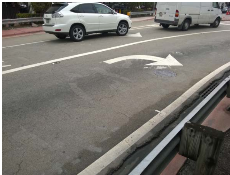
Figure 2.16 – Random cracking likely from thermal incompatibility (Miami Beach-SR A1A)
