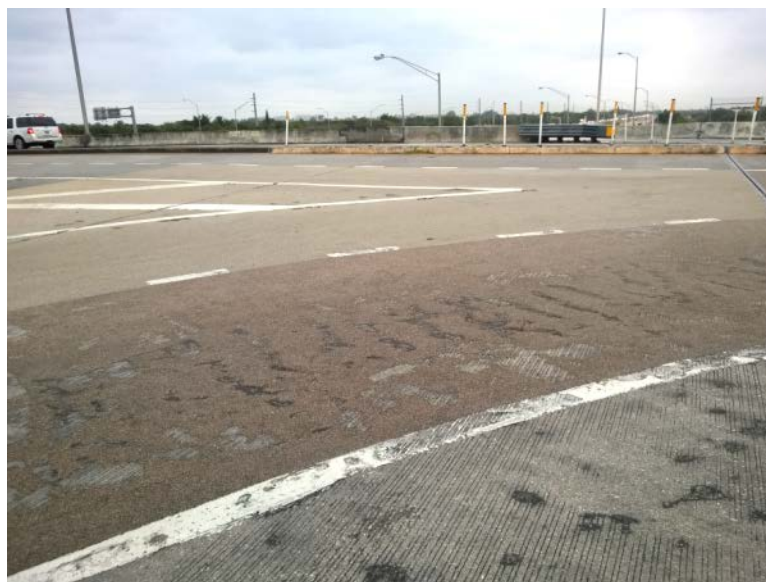
Figure 2.7 – Aggregate loss over concrete, single HFST application (I-95 to Congress)
