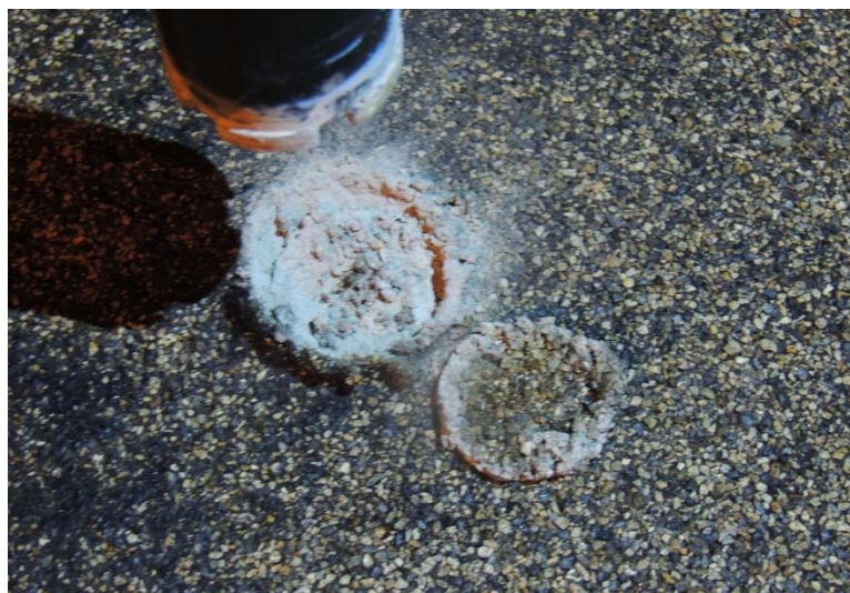
Figure C.17 – Weak bond of splotchy area.
