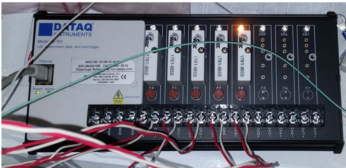
Figure 6-3: The DI-161 Board with Wires and Connections
