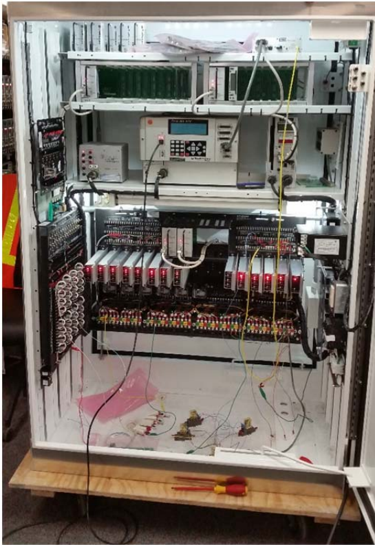
Cabinet with Controller & Loop Detectors
