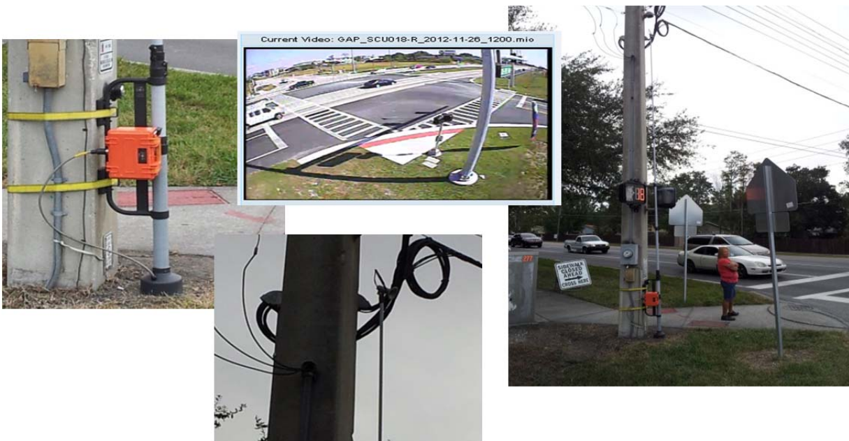
Figure 2-1: VCU Attached to a Utility Pole at a Height of 20 Feet
