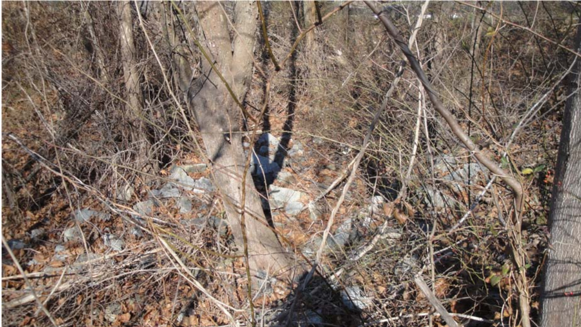
Figure 3. BMP Site # 030189 (US 1), SHA rated IV/Failed. Note: Trees growing along the conduit of the system with intense vegetative cover (all included photographs were taken: Fall/December 28, 2014).
