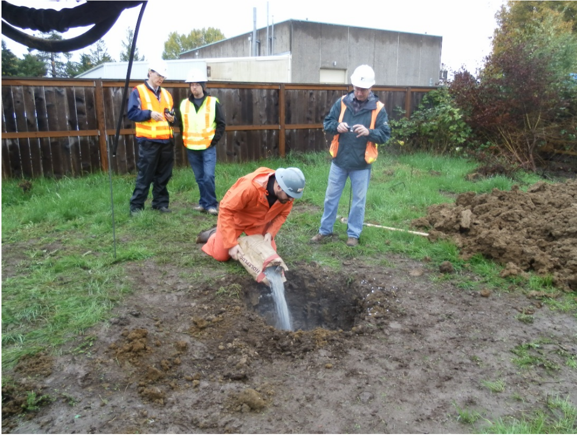
Figure 4.11: Placing bentonite chips at the bottom of excavation of TDSFB following clean-out
