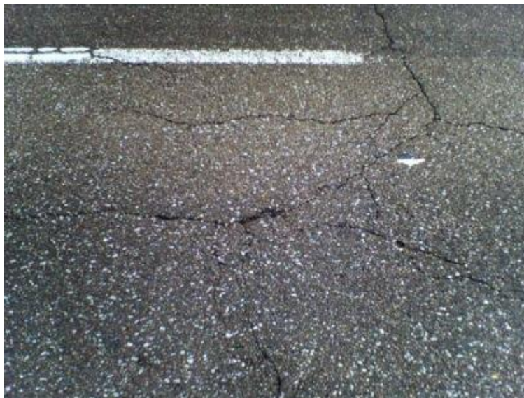
Figure 4.2 Typical Longitudinal Cracks in Pavement
