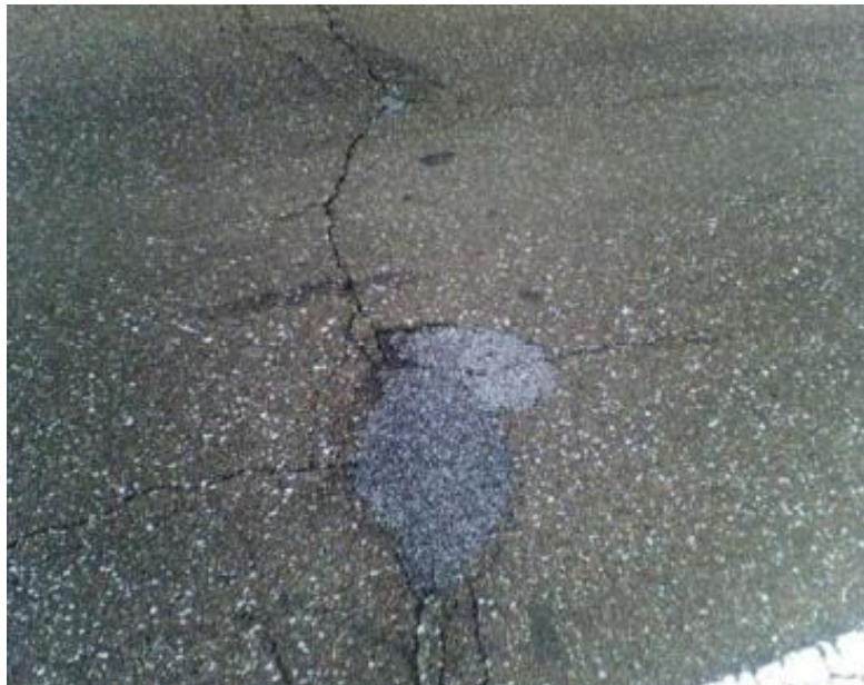
Figure 4.1 Typical Longitudinal Cracks in Pavement
