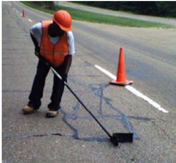
Figure 7.4.3 Cracks Over-Sealed in Sealed Section
