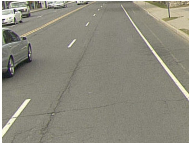
Figure 1. Longitudinal Joint Opening
