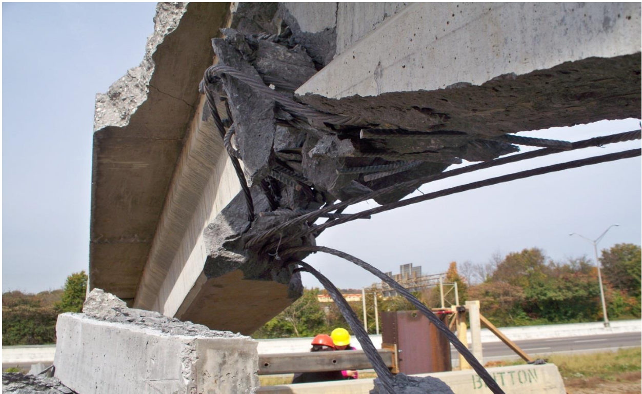
Figure 32. Prestressed beam after impact.
