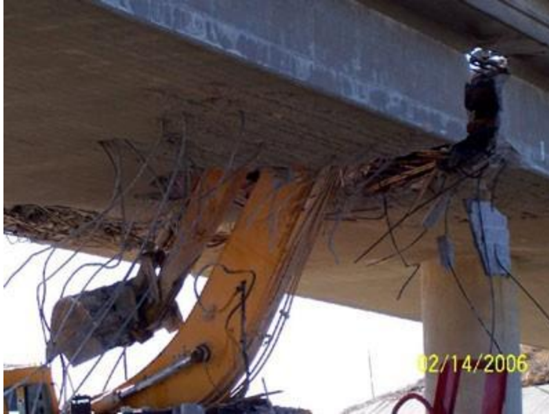
Figure 1. Excavator that has impacted the side of a bridge. (DailyCognition, 2013)
