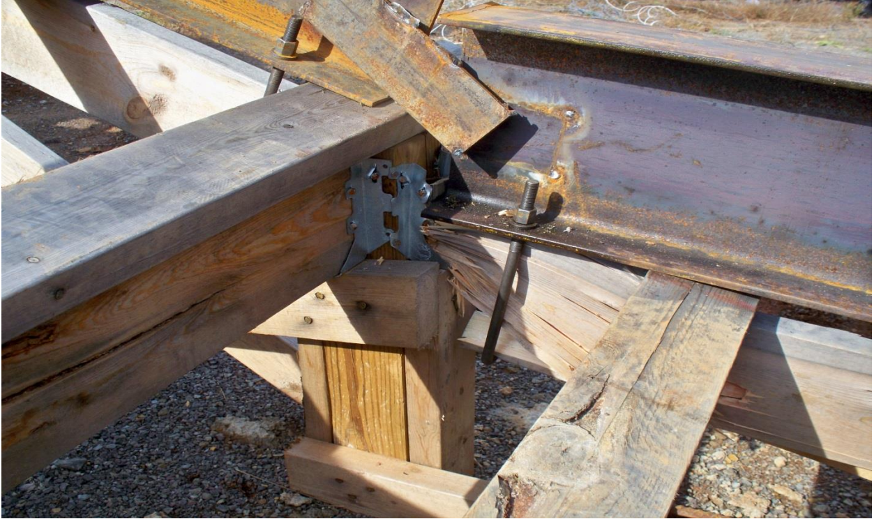
Figure 33. Damage to joists after testing.
