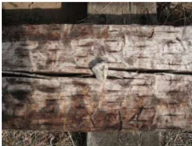
Figure 2.3 Underside of a conventional wood tie removed from service showing indentations from ballast particles. (FRA Task Order 225)
