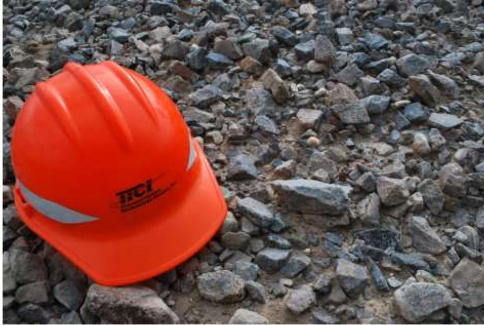
Figure 1.3 An example of fouled ballast
