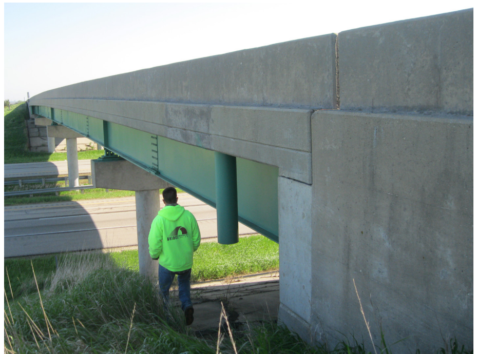
One of the five bridges, the short-span steel girder bridge, that the researchers instrumented and used for load testing
