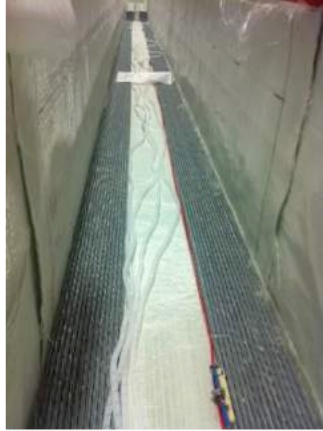
Figure 8 - Internal VWG Placement at Tension Level
