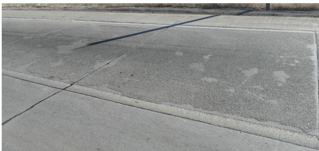
High Friction Surface Location Showing Wear
