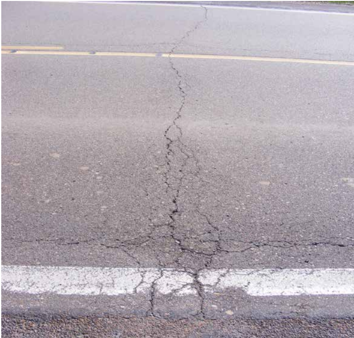
Figure 1.3: Low-Severity Transverse Cracking on US-83 in Thomas County, KS
