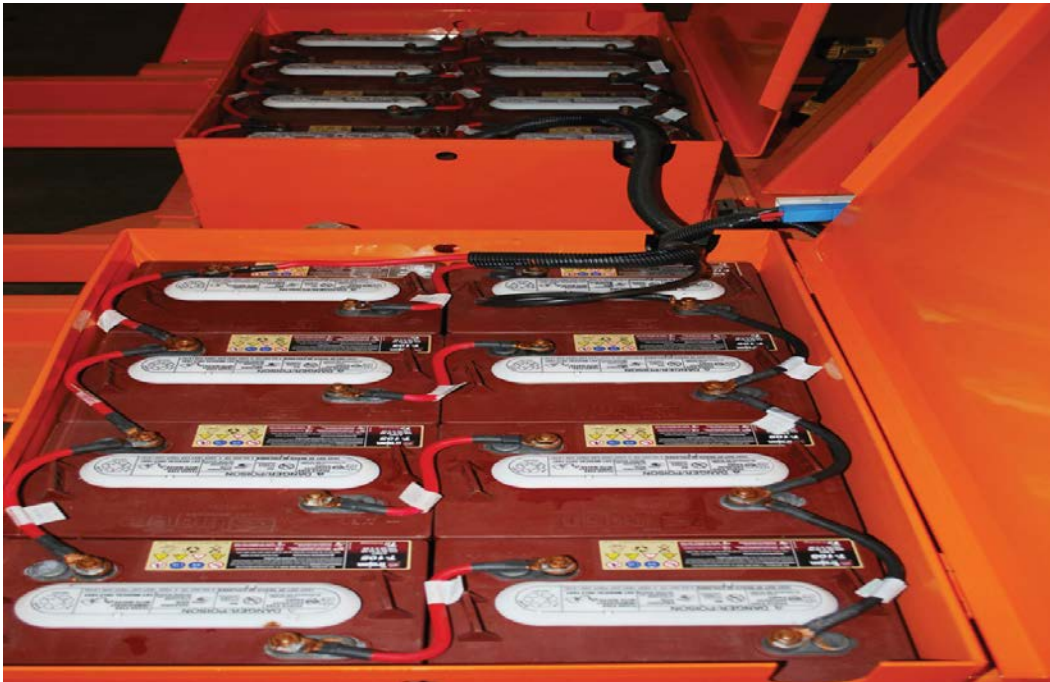
Figure A.4: Batteries Provided (Source: Procurement Specifications PTS-2000)
