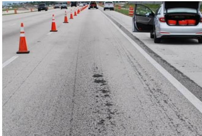
Figure 3-2. Pavement distress observed on I-75 between Sheridan Dr. and Miramar Dr.
