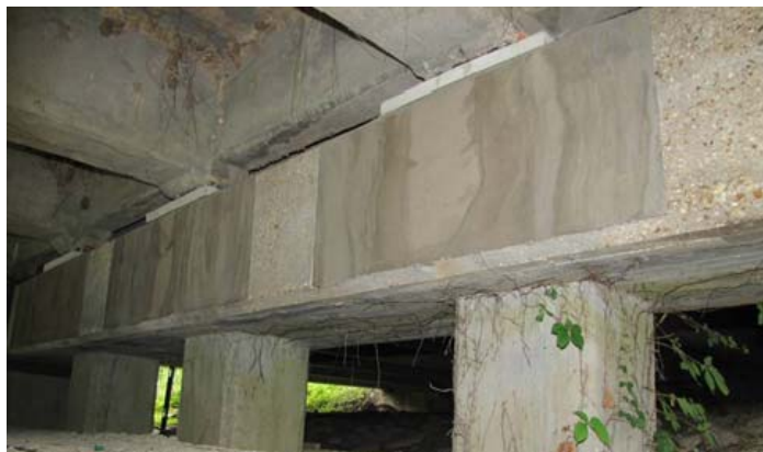
Figure 2 View of the bent after the initial repair: Note the base plates under the beams and the repair material that replaced delaminated concrete
