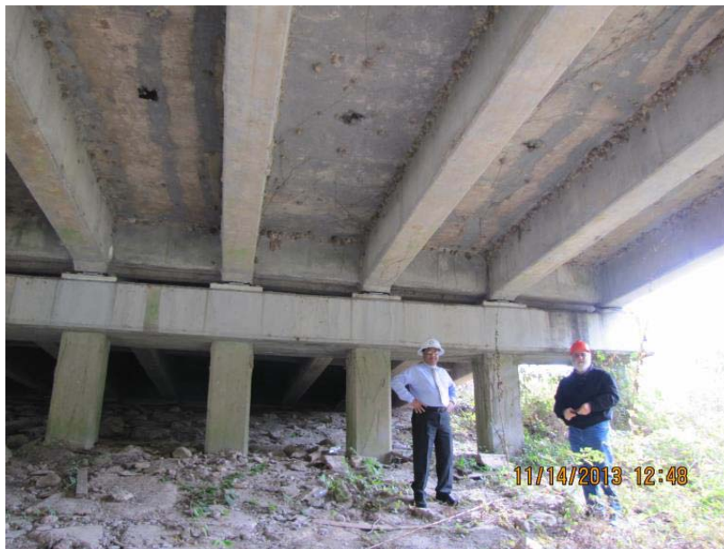
Figure 33 Overall view: Note the debris buildup on the un-coated right side of the structure
