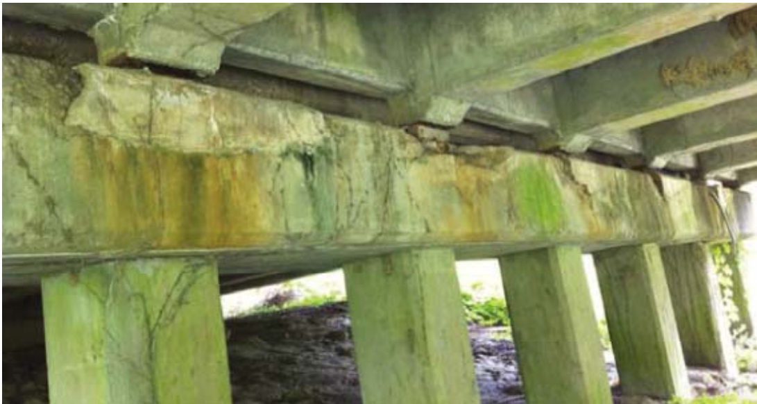
Figure 1 Pier cap pre-repair: Delamination under the bearing plate
