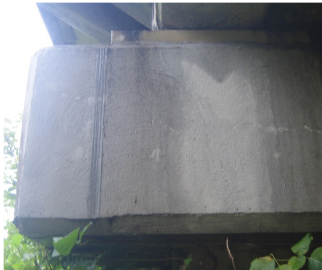
Figure 35 View of high modulus confinement composite: Continuous carbon tows can be seen next to the bearing plate
