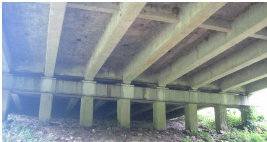
Figure 38 Overall view: Note the debris buildup on the un-coated right side of the structure
