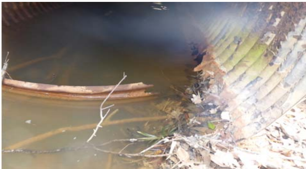
Corroded metal pipes
