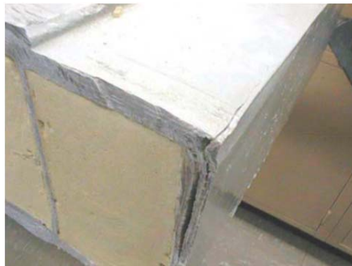
Figure 2: Voids resulting in surface cracks (Ryan et al [3])
