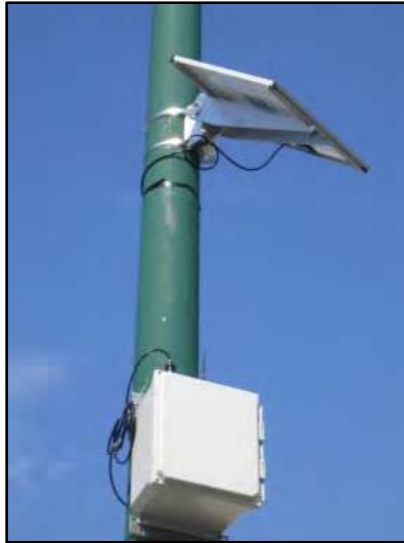
Figure 3 Bluetooth device mounted on a light pole
