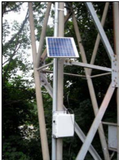
Figure 4 Bluetooth device mounted on a truss
