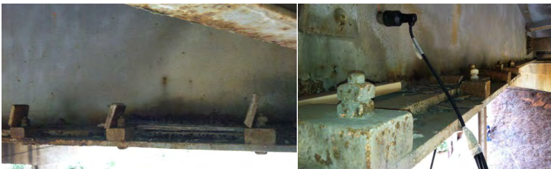
Figure 30. 3 of 4 broken plate clamps (left) and an undisturbed setup on Beam 2 (right).
