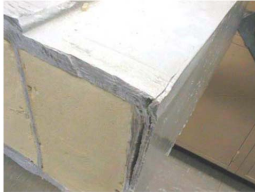
Figure 1: Voids resulting in surface cracks (Ryan et al [1])
