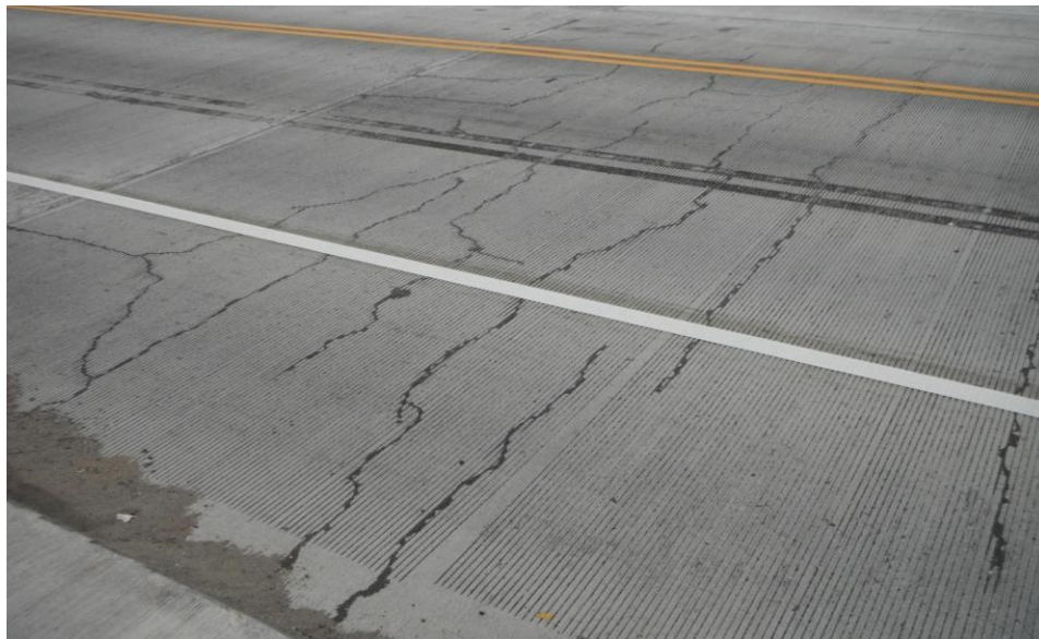
Figure 3. Transverse Cracks on Route 61 Over New River (Salem District)
