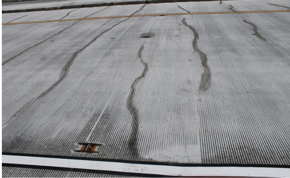
Figure 2. Transverse Cracks on Nimmo Parkway (Hampton Roads District)
