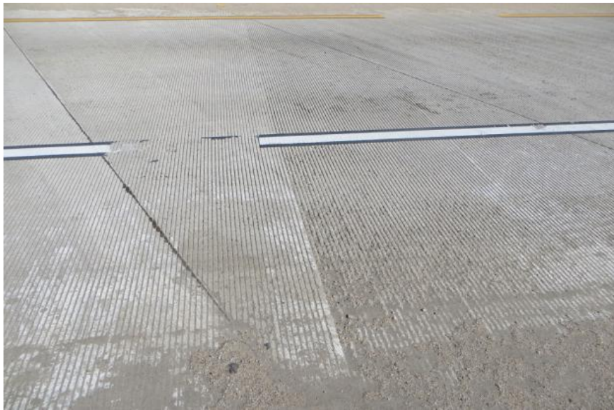
Figure 7. Scaling at Closure Pour of Route 15 Opal Bridge at Lower Middle Portion of Photograph
