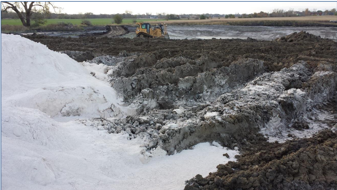
Figure 6. Wet unstable areas of fill that required lime stabilization, and load of lime ready for incorporation into soil
