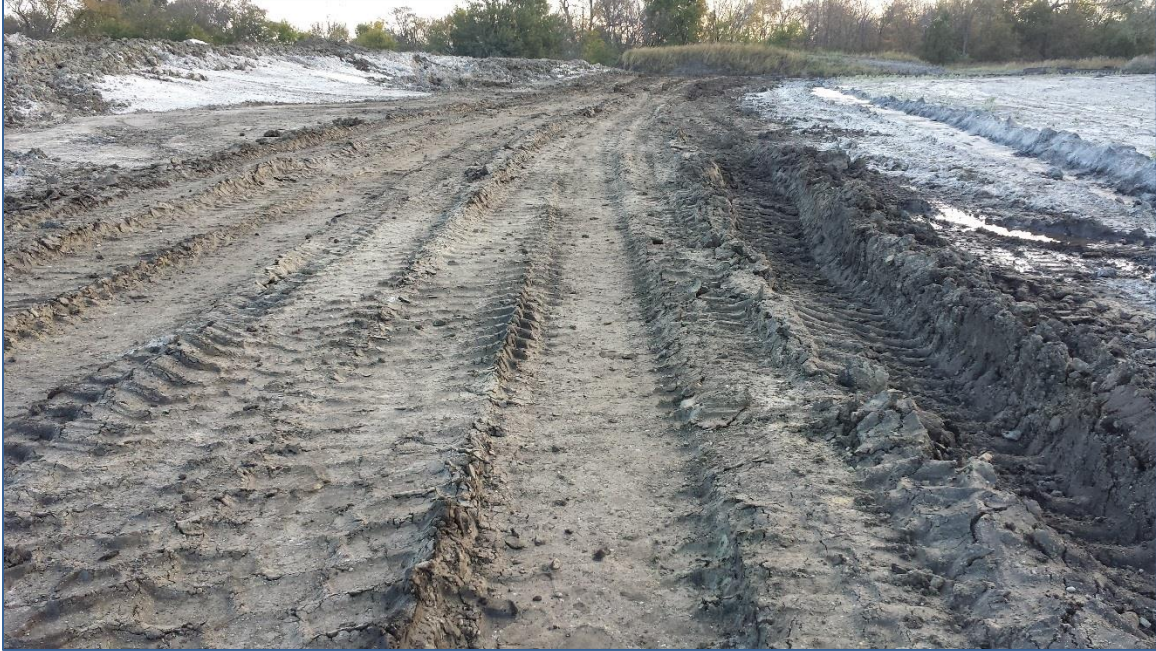
Figure 7. Section of haul road observed to pump and rut under haul truck operations
