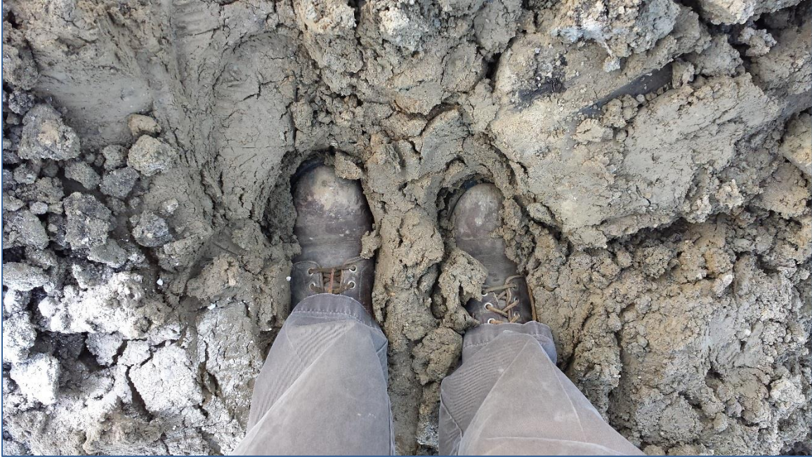
Figure 5. Wet unstable areas of fill that required lime stabilization
