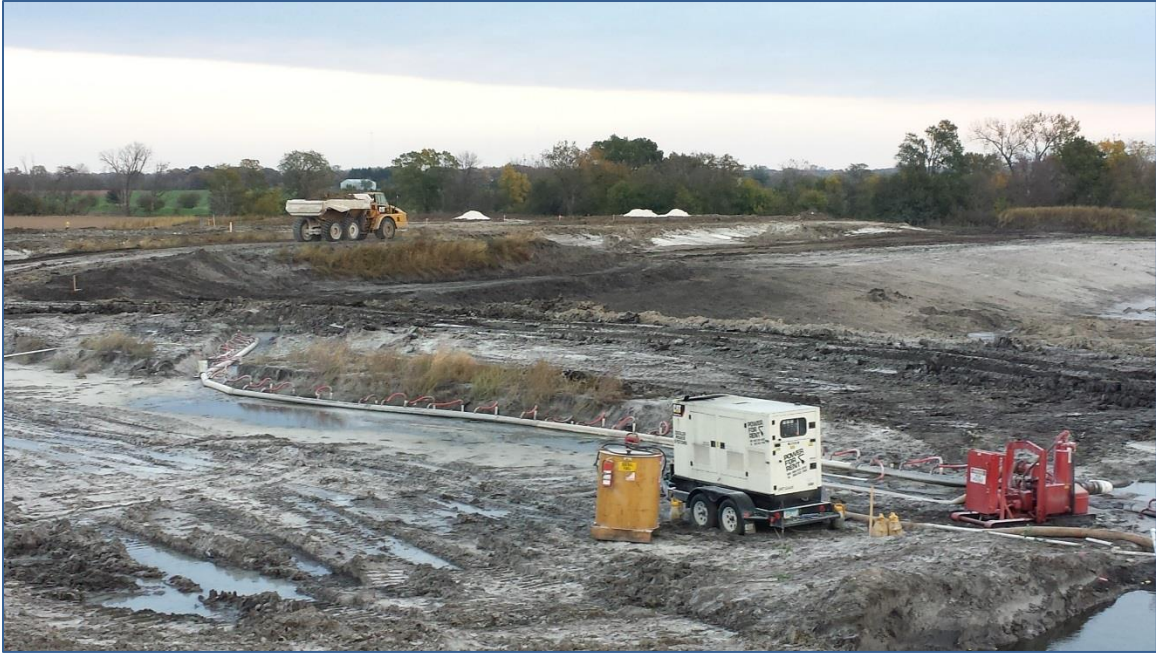
Figure 11. Dewatering operation for pond area and loaded haul truck on haul road
