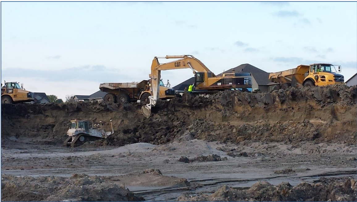
Figure 8. View from bottom of pond area showing the area being excavated and loaded into haul trucks
