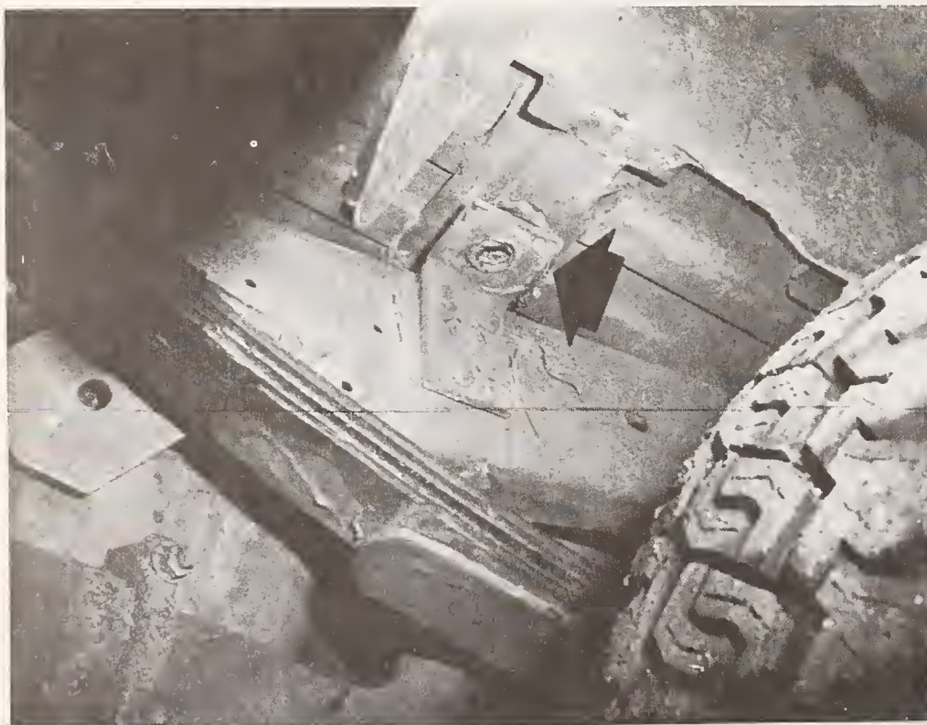
The TECHNICIAN TRAINING SCHOOL , McKees Rocks, Pennsylvania, forwarded to the PRP the photo shown above. The arrow indicates a missing frame bolt on the left rear of a 1978 Plymouth Trail Duster. According to the school, the vehicle was delivered with three out of the four front frame bolts missing and three out of the four rear frame bolts missing. The problem was reportedly noticed when the vehicle was taken out of service because of adverse body sway.
