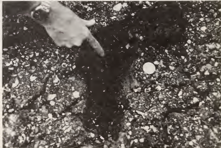
b. Closeup showing separation of lifts and moisture within asphalt stabilized shoulder.
