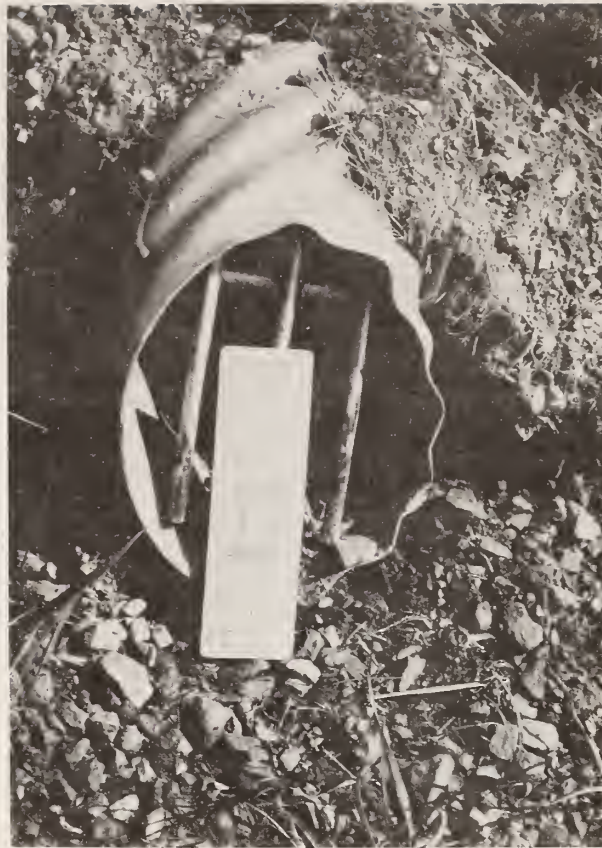
Figure 6.13. Corrugated Metal Subdrain Outlet Pipe in Canada.
