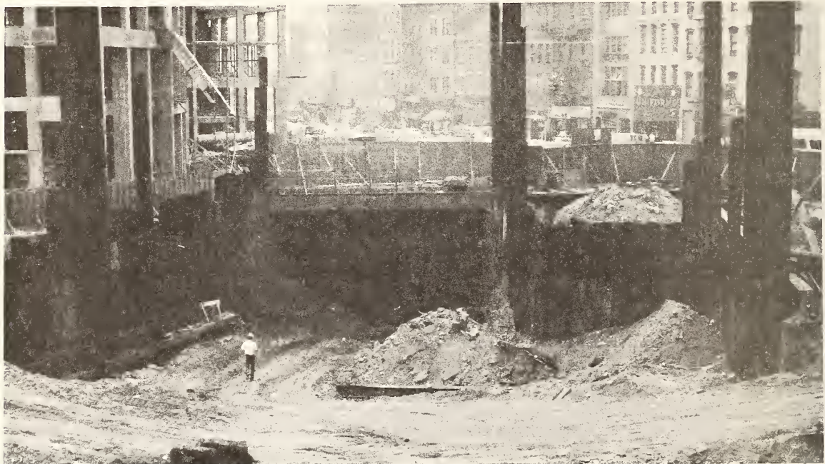
Figure 36. Sheet piling on obstruction missed in site investigation.
