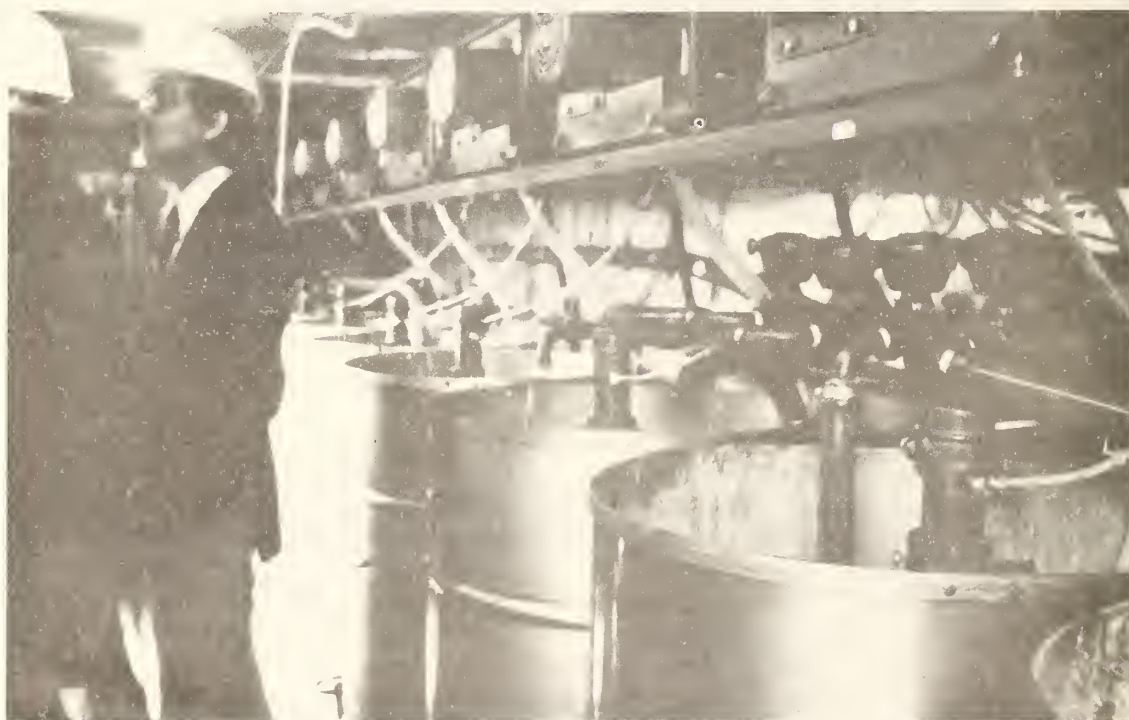
Figure 51. Grout pumps and mixing tanks in van unit.
