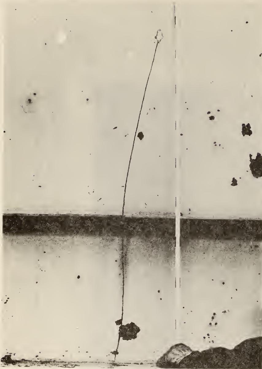
Figure 5-20 Crack in web of Fascia Girder.
