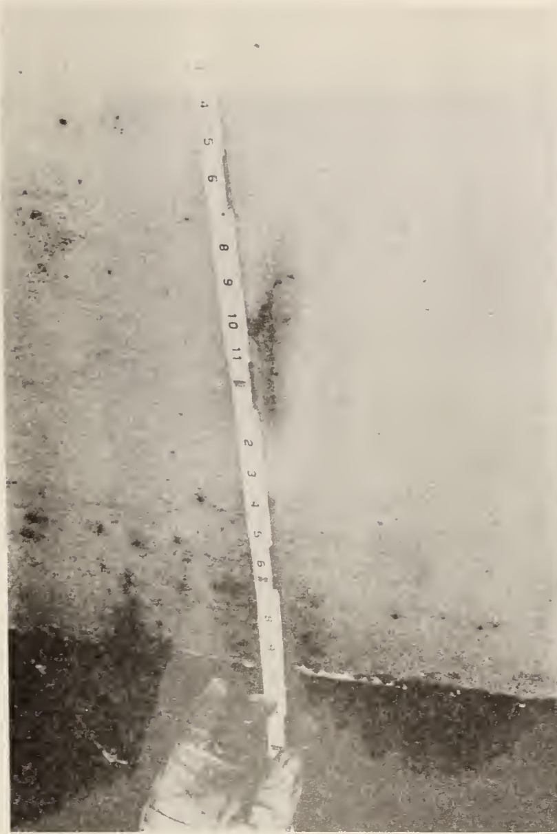
Figure 5-21 Crack on bottom of beam flange.
