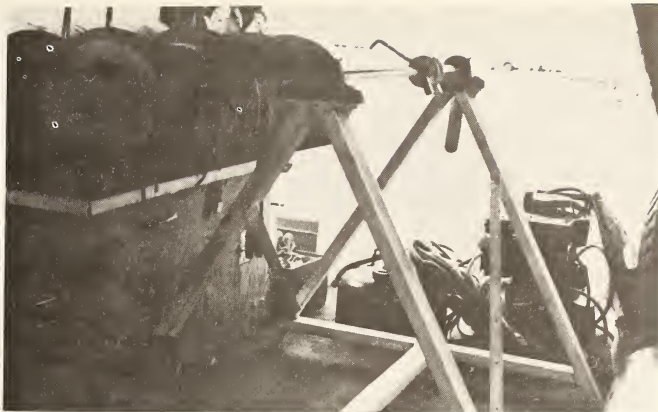
Figure 74. Lead-in cables and electrical generator.
