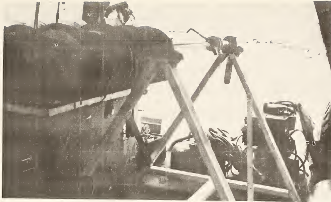
Figure 30. Lead-in cables and electrical generator.
