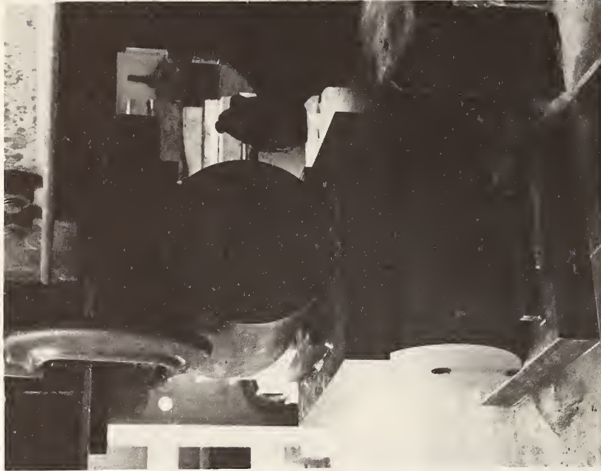
(b) Support at Joint 2, Showing Short Blocks Which Allow Both Rollers to Move Freely
