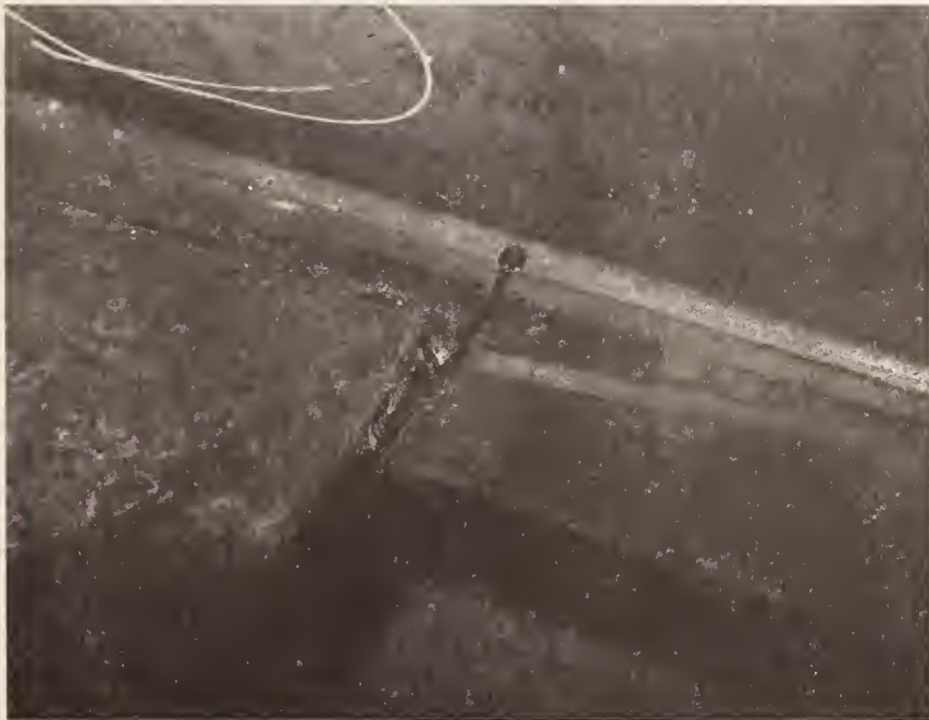
Fig. 59 Typical Fatigue Cracks - Details V_{oa} and V_{ob}
