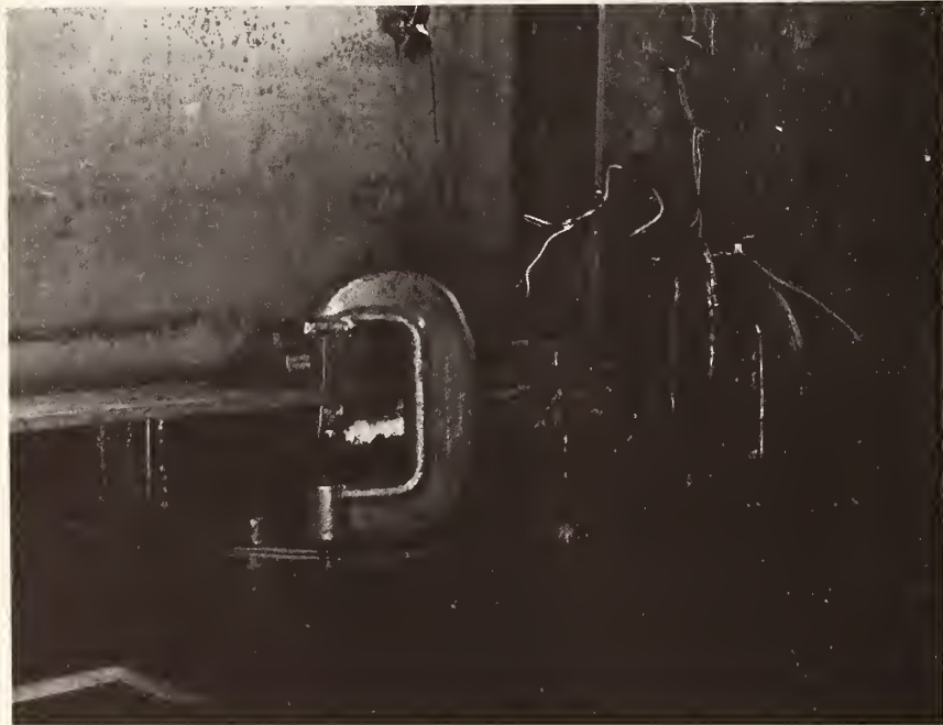
Fig. 52 Typical Flange Crack Repairs - Drilled Holes at Type V o Detail - Splice Plates Clamped to Flange
