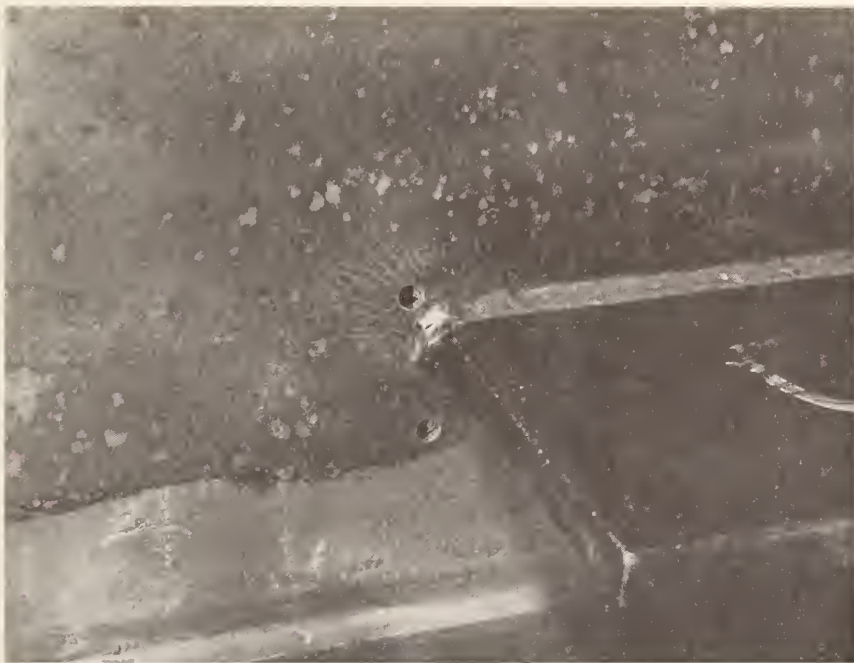
Fig. 51 Typical Web Crack Repairs - Drilled Holes at Type II o and III ob Details
