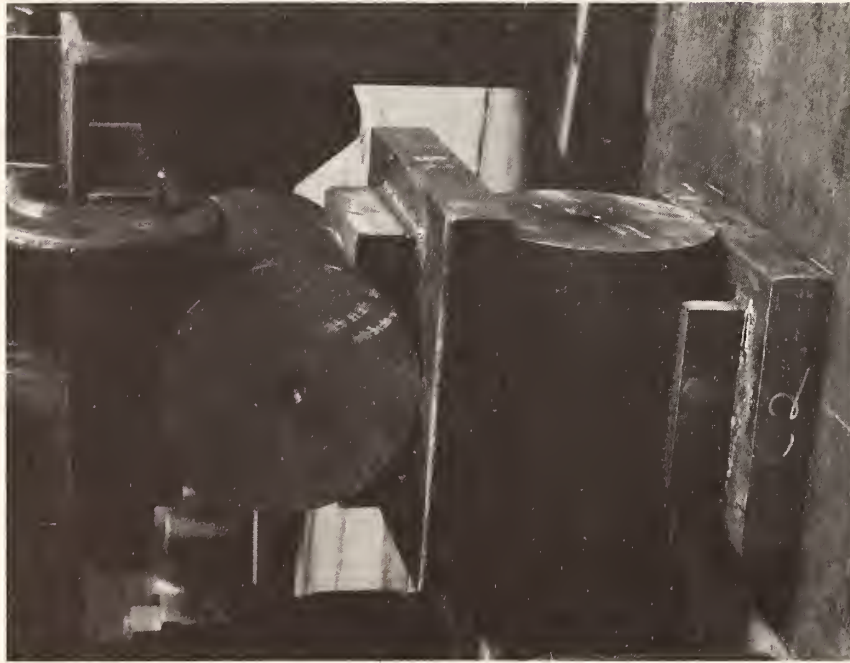
(a) Support at Joint 1, Showing High Blocks Which Prevent Radial and Tangential Motion
