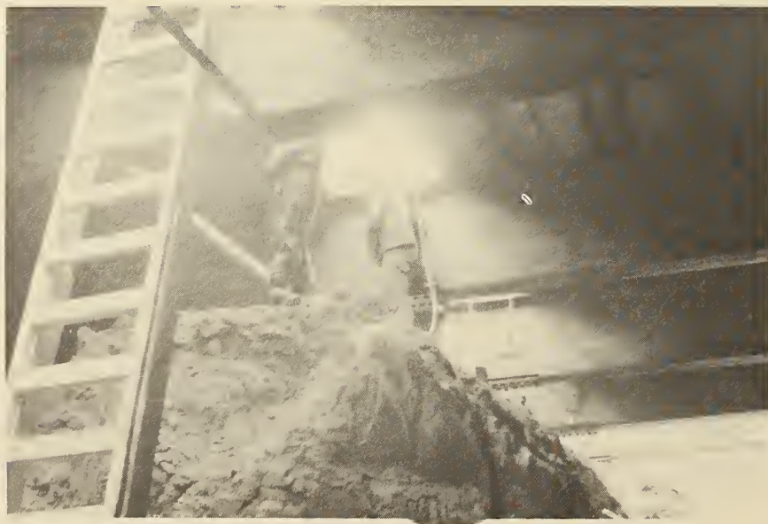
FIGURE 47. TORONTO SUBWAY, Installing and Splicing the Deck Beams. The half-section of the tunnel on the left side of the picture is already decked, and decking is in progress on the right side. The soil in the middle is supporting the deck beams. The soil was removed when the deck beams were spliced with bolts.
