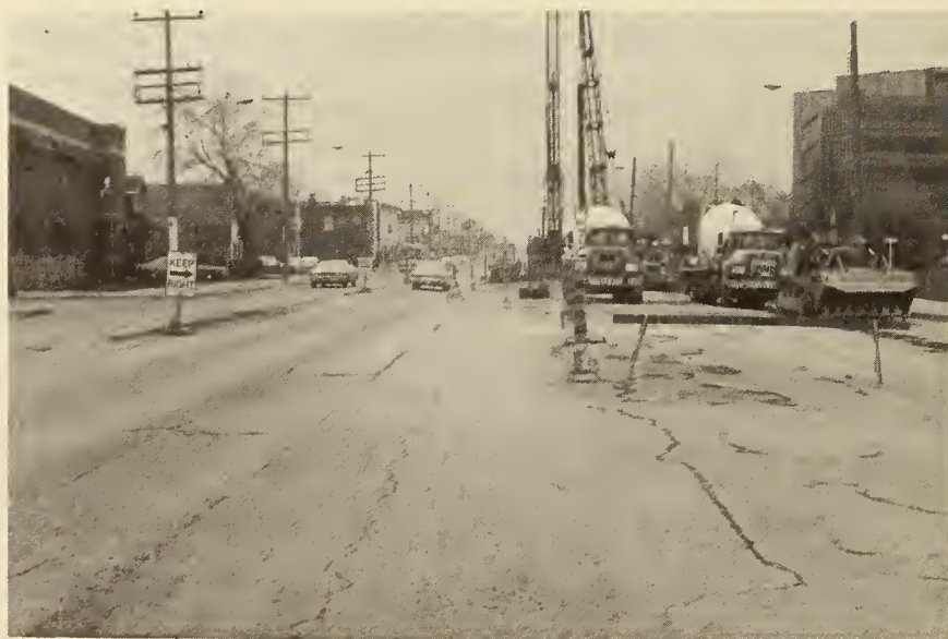
FIGURE 112. TORONTO SUBWAY, YONGE STREET AFTER RESTORATION, looking south. Overall view of method of installing the soldier piles and how the traffic was rerouted. Note the locations in the foreground where the soldier piles were installed; the pavement has been restored.
