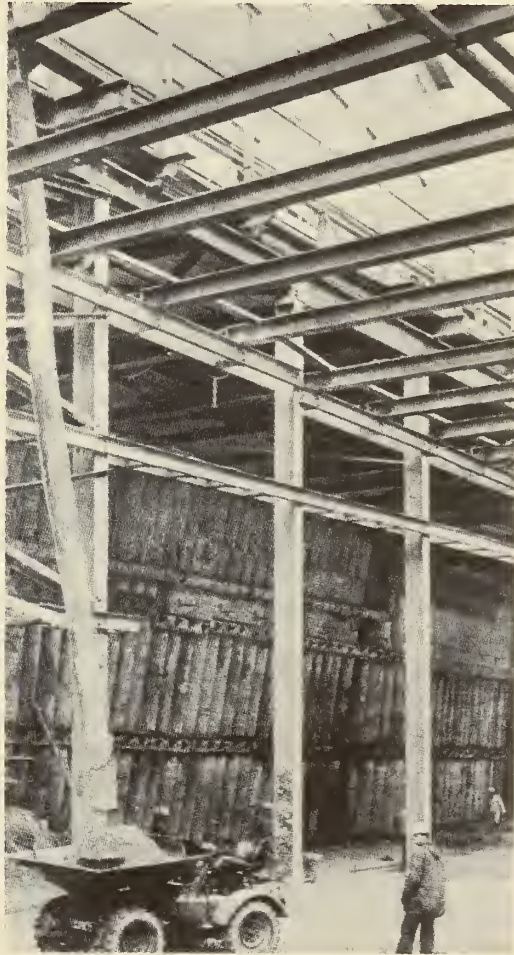
FIGURE 109. MUNICH, GERMANY, INCLINED PILE WALLS protect a department store against a deep excavation. The wall is braced at the top, and it is tied back below by two rows of anchors grouted into the earth and prestressed. (From Civil Engineering , July, 1970, p. 67, by permission.)
