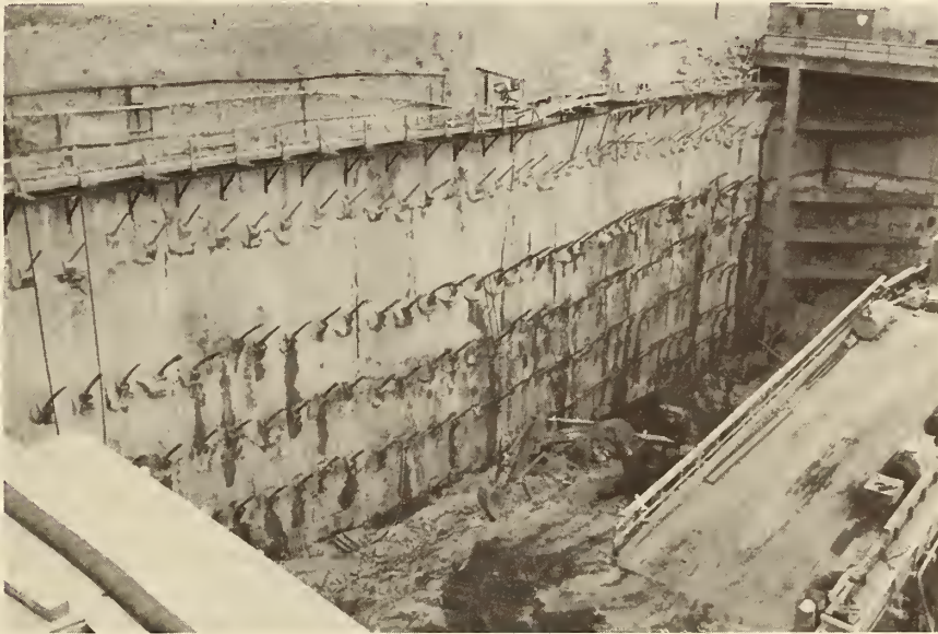
FIGURE 77. SLURRY-TRENCH WALL FOR BANK BUILDING in Stockholm. One adjacent multistory brick building (upper part of wall in picture) settled two inches during excavation.
