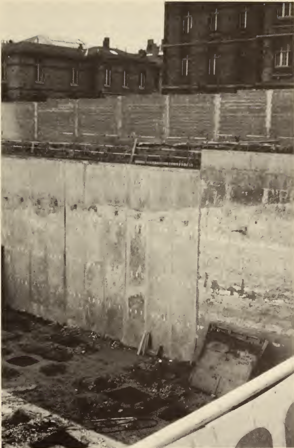
FIGURE 103. JUNCTION BETWEEN PRECAST AND CAST-IN-PLACE SLURRY WALLS, both built in a slurry trench, Paris. Note the tiebacks and styrofoam-filled pockets for the concrete floorbeams.
