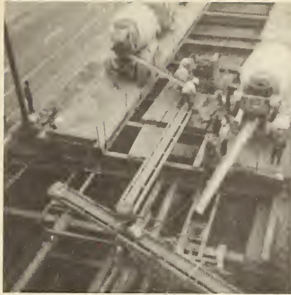
FIGURE 55. ACCESS DECK DISCONTINUITY (Courtesy of Fruin-Colnon Contracting Company.)
