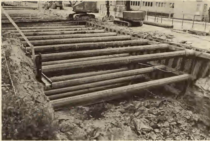
FIGURE 26. EXCAVATION FOR SUBWAY ENTRANCE AT OLAF KYRRES PLACE, Oslo, showing cross-lot braced sheet piles.
