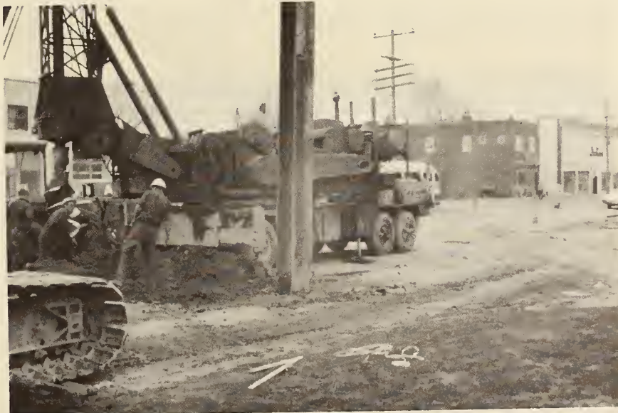
FIGURE 18. TORONTO SUBWAY, Soldier-Pile Drilling Operations. The Contractor was having trouble augering through a boulder. The soldier pile in the foreground was used to break the boulder.
