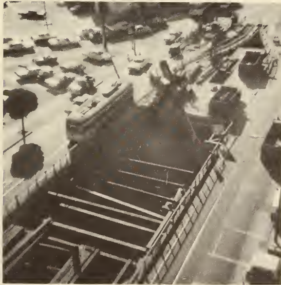
FIGURE 56. EXCAVATING BEYOND PLATFORM at the west end of the job where the shoofly tied into the existing tracks. (Courtesy of Fruin-Colnon Contracting Company.)
