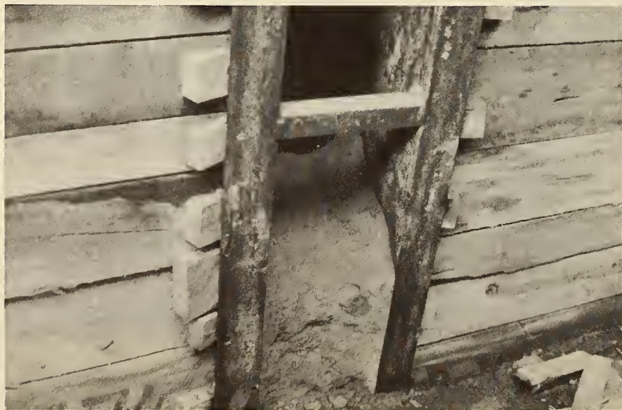
FIGURE 20. TORONTO SUBWAY SYSTEM, Wall-Support System. A close-up of a soldier pile, timber lagging, and the wedging system. The material between the flanges of the soldier beam is lean concrete.
