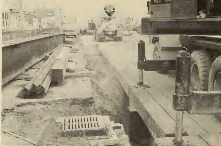
FIGURE 46. TORONTO SUBWAY, Seating the Timber Decking. A lean concrete was used to backfill behind the lagging and up to the timber decking. The lean concrete was then capped with 6 inches of 3,000-psi concrete.
