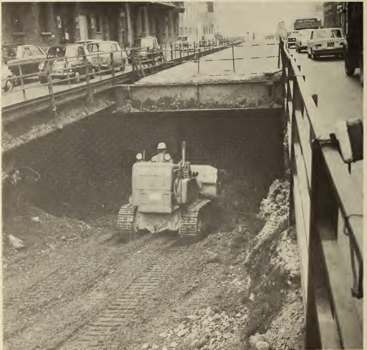
FIGURE 96. EXCAVATION BETWEEN SLURRY WALLS, Milan, Italy. (By permission of ICOS Corporation of America.)
