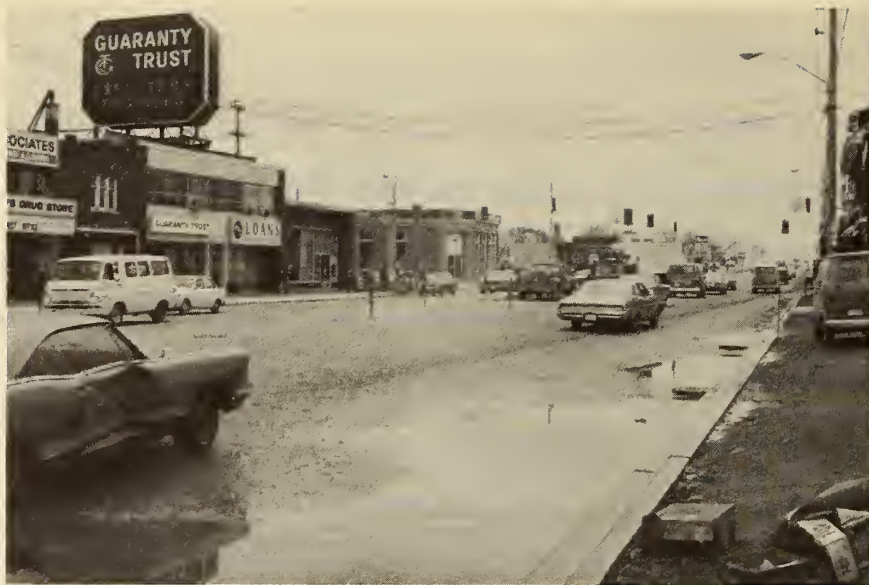
FIGURE 111. TORONTO SUBWAY, YONGE STREET AFTER RESTORATION, looking south. Restoration is almost complete. The station is located to the right out of view. The standing water in the foreground shows where the Contractor had settlement problems.
