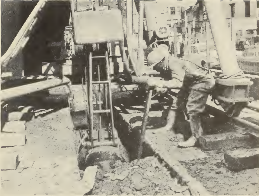
FIGURE 84. WORLD TRADE CENTER, NEW YORK, Slurry-Trench Excavation Using the ICOS-Icanda Method. (By permission of ICOS Corporation of America.)
