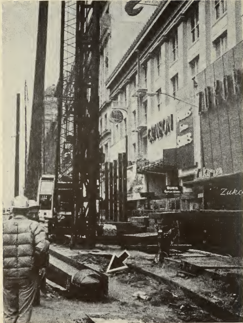
FIGURE 92. BART, SAN FRANCISCO, Soldier-Pile Tremie-Concrete Method (SPTC), Soldier Beams with Driving Shoes. (From Engineering News-Record , July 11, 1968, p. 44, by permission.)
