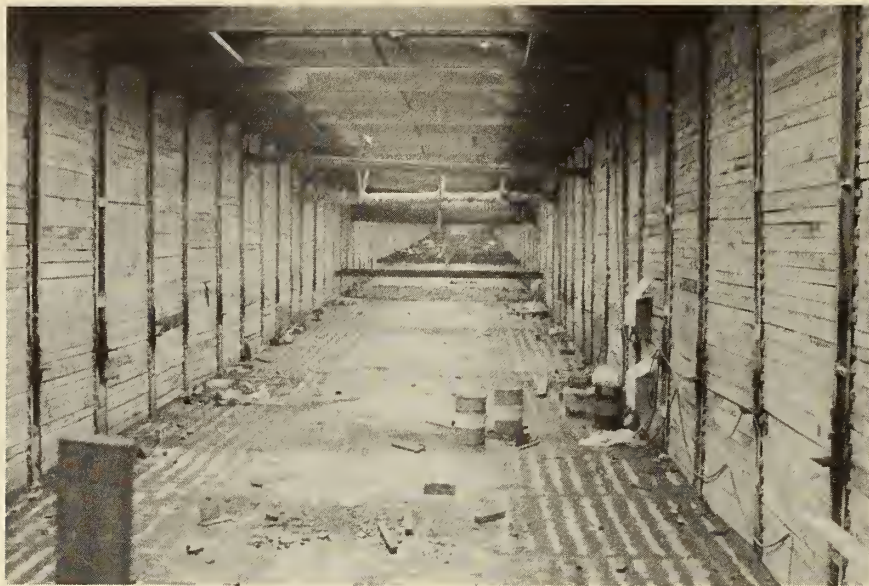
FIGURE 19. TORONTO SUBWAY, Yonge Street Construction, looking north along the subway below Yonge Street. The space in the picture is between the roof of the subway and the street. Utilities can be seen hanging from the deck beams in the middle of the picture. The soldier piles in this location are two channels and not the usual I-beams. Lagging has been wedged against the soil. The light area in the upper part of the picture is from an opening in the decking. Two struts have been used in this section, the deck beam at the top, and the strut immediately above the roof of the subway. Foreground--the strut above the roof has been removed.
