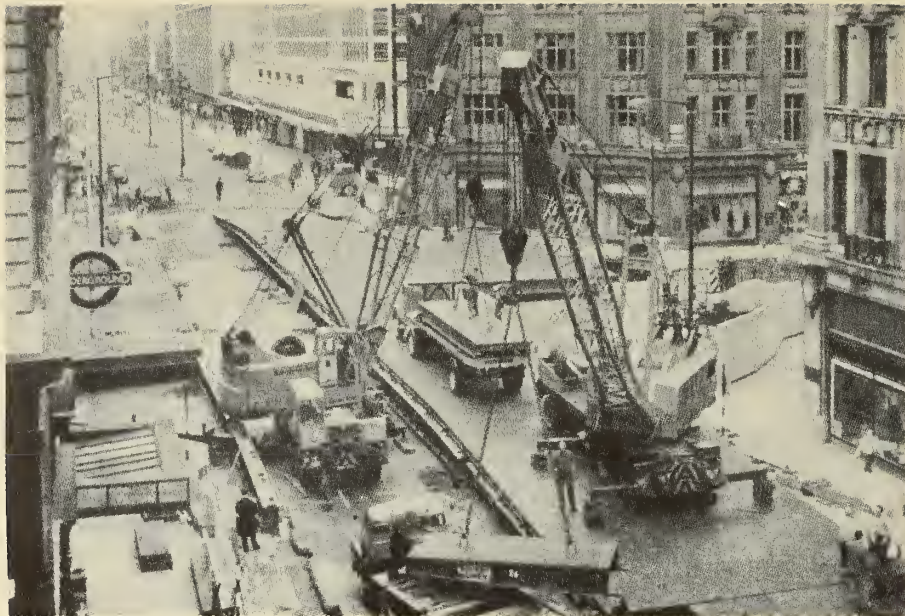
FIGURE 60. UMBRELLA DECKING, LONDON. Subsurface construction under busy streets can be done by covering the surface with temporary bridging. This busy intersection was completely covered during the weekend with an "umbrella" of steelwork panels complete with road surfacing. A ticket hall concourse was constructed under the temporary work, and the busy road traffic was carried without interference.
