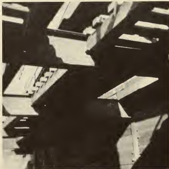
FIGURE 58. 33 WF DECK BEAMS and 14-inch square timber supports the Muni Railroad at the west end of the job. (Courtesy of Fruin-Colnon Con- tracting Company.)
