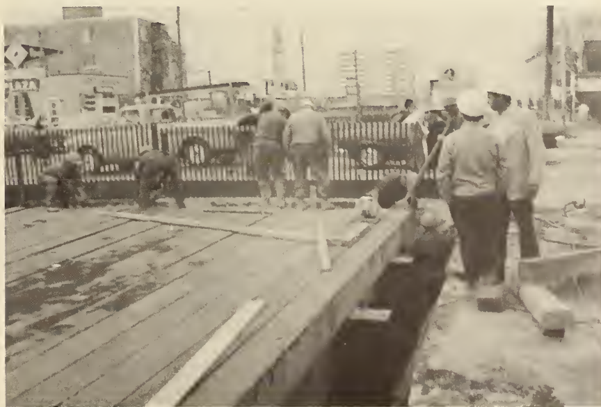
FIGURE 49. TORONTO SUBWAY, Decking Installation, looking north along Yonge Street. The workers are installing timber decking. Only a quarter of the intersection was taken out of service at any one time. This picture does not show the policeman directing the traffic (two directed traffic during the rush hour).
