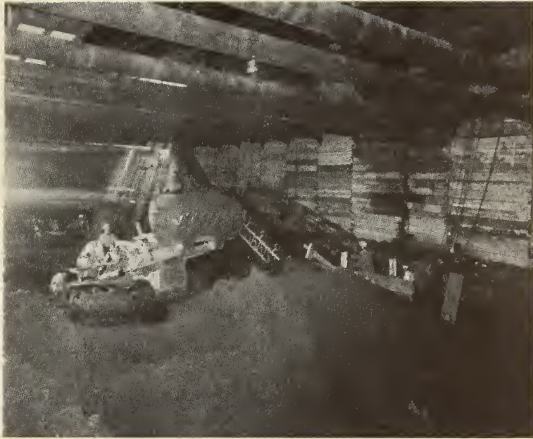
FIGURE 44. BART, SAN FRANCISCO, Spoil Removal by Conveyor. (From Engineering News-Record , July 24, 1969, p. 30, by permission.)
