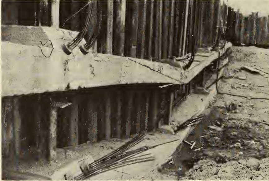
FIGURE 23. CONCRETE WALES CAST ON THE GROUND, directly on the excavation bottom. Friction-reducing cardboard is inserted between the concrete and the sheets. The procedure of driving sheets, excavating, tying-back the soldier piles and casting the concrete waler is repeated until bedrock is reached.
