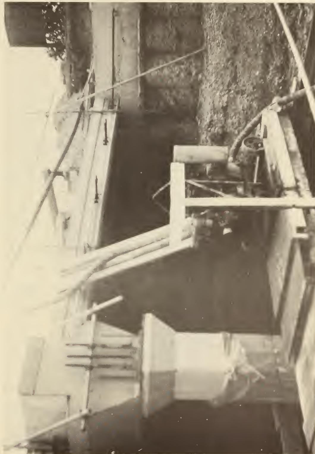
FIGURE 107. EXPOSED WALLS OF CONTINUOUS BORED-PILES, London, England. A precast roof structure post-tensioned longitudinally is also shown.
