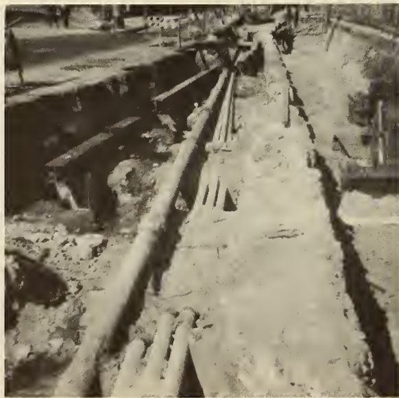
FIGURE 54. SOLDIER PILES AND CAP BEAMS. Live water lines and two live telephone ducts were to be supported. (Courtesy of Fruin-Colnon Contracting Company.)
