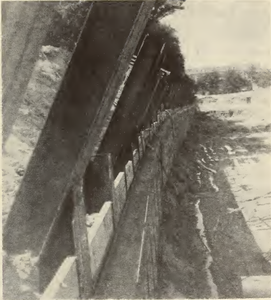
FIGURE 28. WASHINGTON, D. C., Soldier Beams Tied-Back with H-piles secure deep excavation. (From Engineering News-Record , October 19, 1967, p. 47, by permission.)
