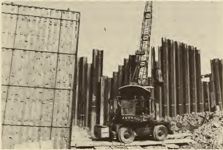
FIGURE 2. STOCKHOLM, SWEDEN, NOISE CONTROL MEASURES NEAR A HOSPITAL. The construction was near a hospital, and rubber caps were put on the sheet-pile hammers. The drill hammers were enclosed and screens (at left in the picture) were placed between the machines and the hospital to reduce the noise.
