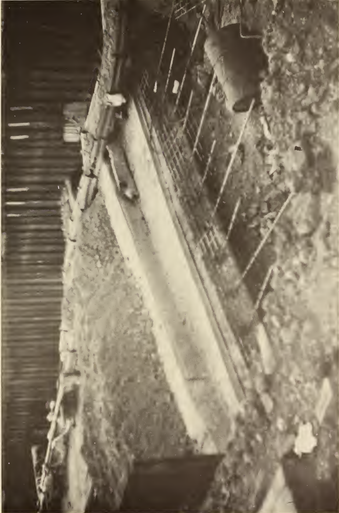
FIGURE 70. PRECAST ELEMENTS USED FOR ROOF OF PICCADILLY LINE extension in London, England. Note the reinforcing bars through the section web. The step marks a change in the roof elevation.
