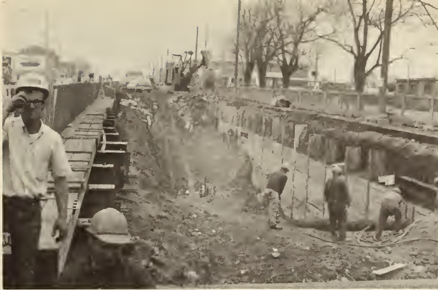
FIGURE 48. TORONTO SUBWAY, Deck Beam Installation, looking south along Yonge Street. The laborers at right are manually exposing an oil line. The ramp to the excavation was previously north of the utilities. The Contractor had to jump over and start a new ramp.
