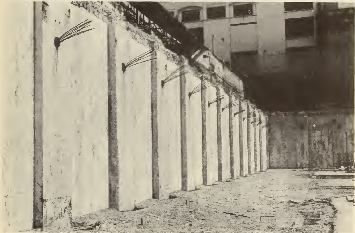
FIGURE 101. WALL CONSTRUCTION BY THE SOLETANCHE METHOD in Paris. Precast elements follow in a slurry trench. (By permission of Soletanche Entreprise, Paris.)
