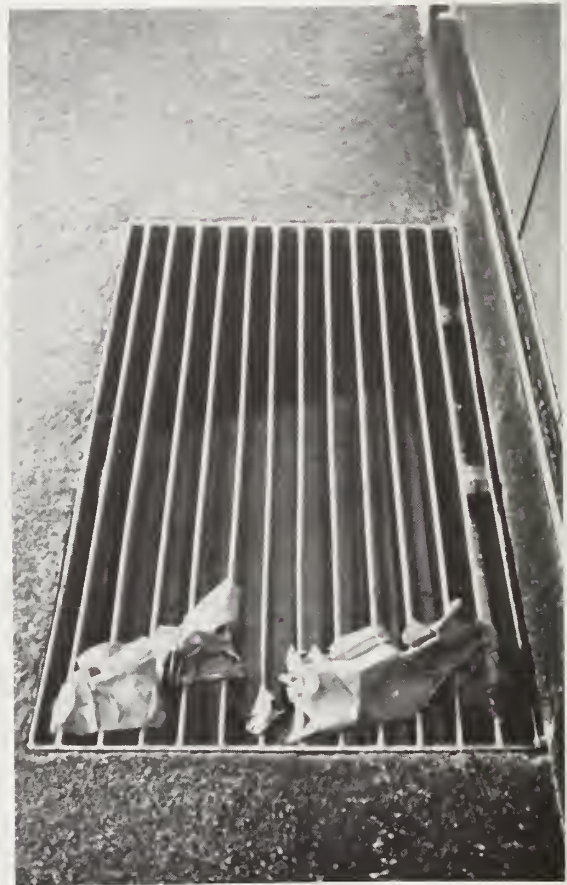
Figure 6-19. - Debris test, 2 ft by 4 ft (0.61 m by 1.22 m) parallel bar grate, S_0 = 4\% , Z = 24 .
