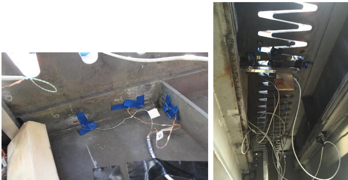
Figure 6-5: Strain gage locations on underside of finger plate expansion device on Blanchette Bridge
