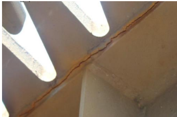
Figure 5-1: Fractured support weld on finger plate expansion device
