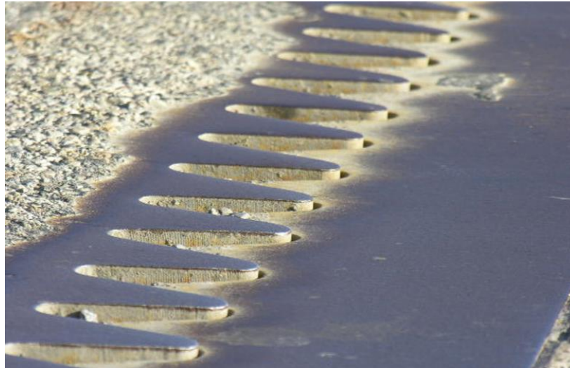
Figure 2-1: Vertical misalignment of finger plate expansion device [2]
