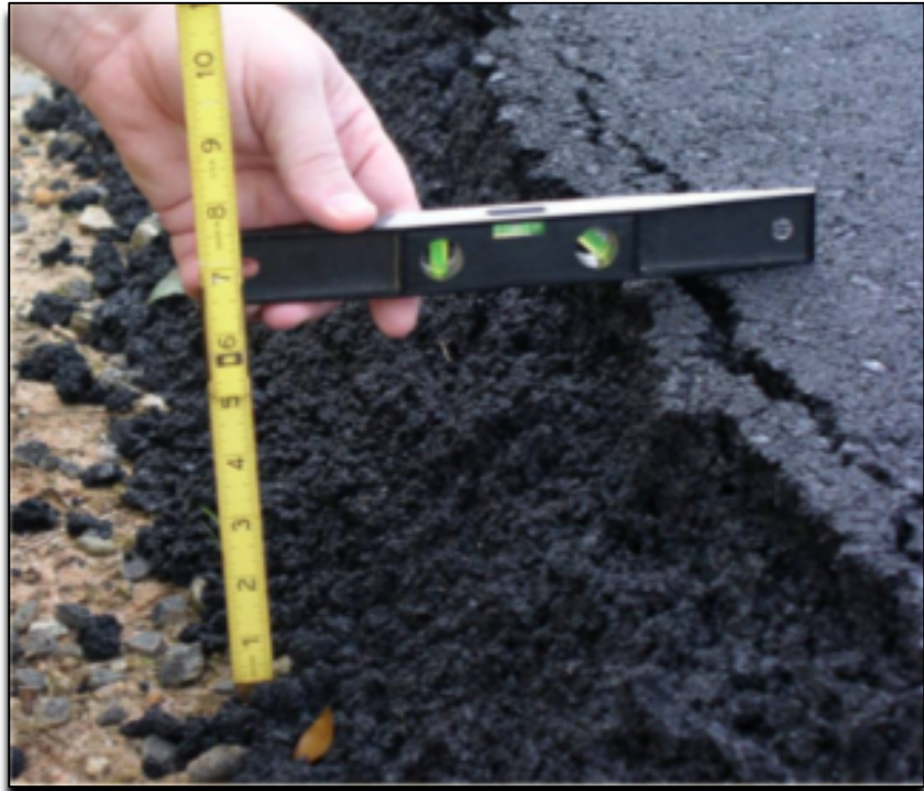
Figure 10: Pavement without Safety Edge
