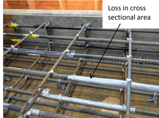
Figure 3.38: Cross-sectional Area loss
