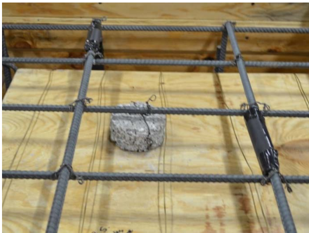
Fig. 3.15: Honeycomb at the top of box beam
