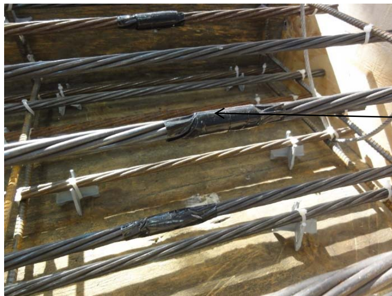
Figure 3.39: Strands showing loss of wires covered with Dual wall polyolefin tube and duct tape
