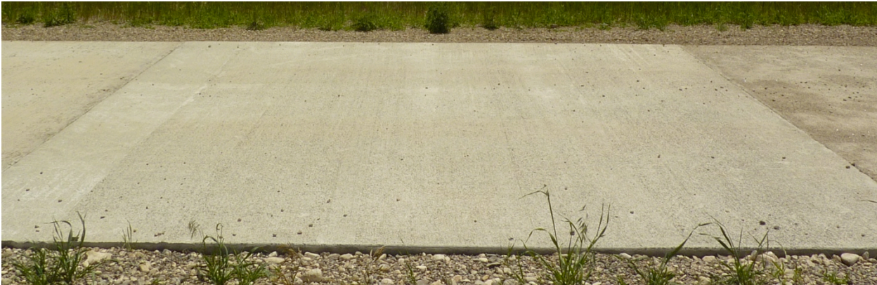
Figure 13: Control Slab at Two Years
