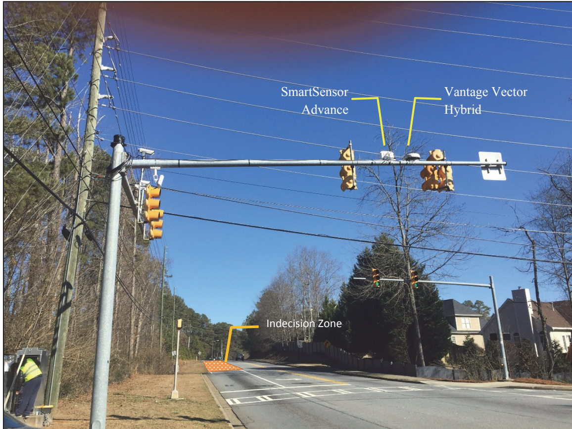
Figure 5.9 Field installation of the advance detection devices for indecision zone detection at site 2
