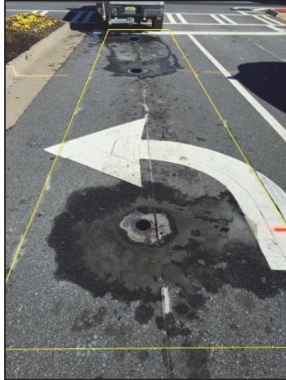
Figure 5.12 Field installation of wireless magnetometers in the northbound left turn lane (site 3)
