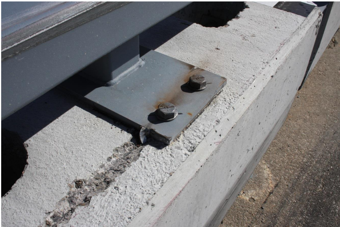
Figure 115. System Damage, First Upper Tube Assembly Connection Upstream from Joint between Barrier Nos. 6 and 7, Test No. SFH-3
