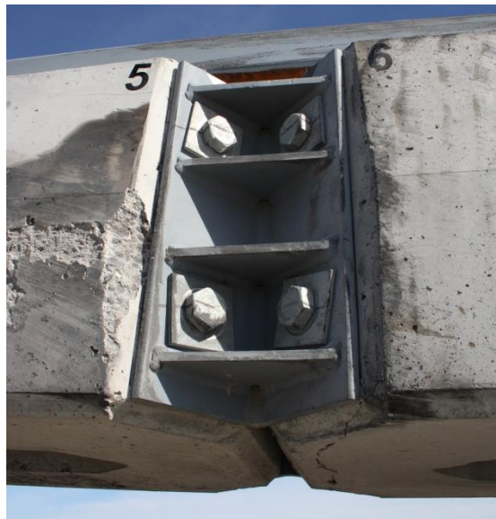
Figure 112. System Damage, Post Contact and Joint between Barrier Nos. 5 and 6, Test No. SFH-3
