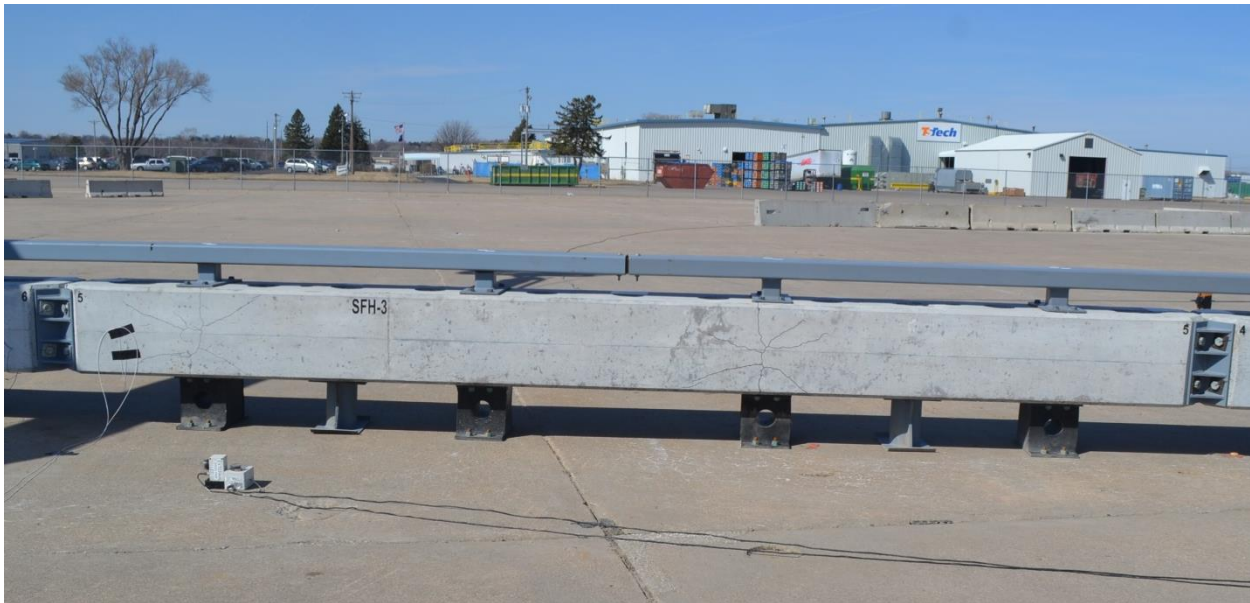
Figure 103. Concrete Beam Cracks Due to Freeze-Thaw
