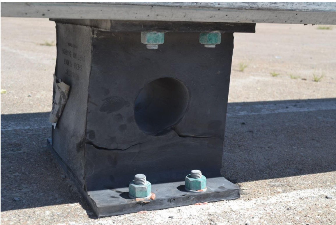
b) Second Post Downstream from Joint between Barrier Nos. 7 and 8
