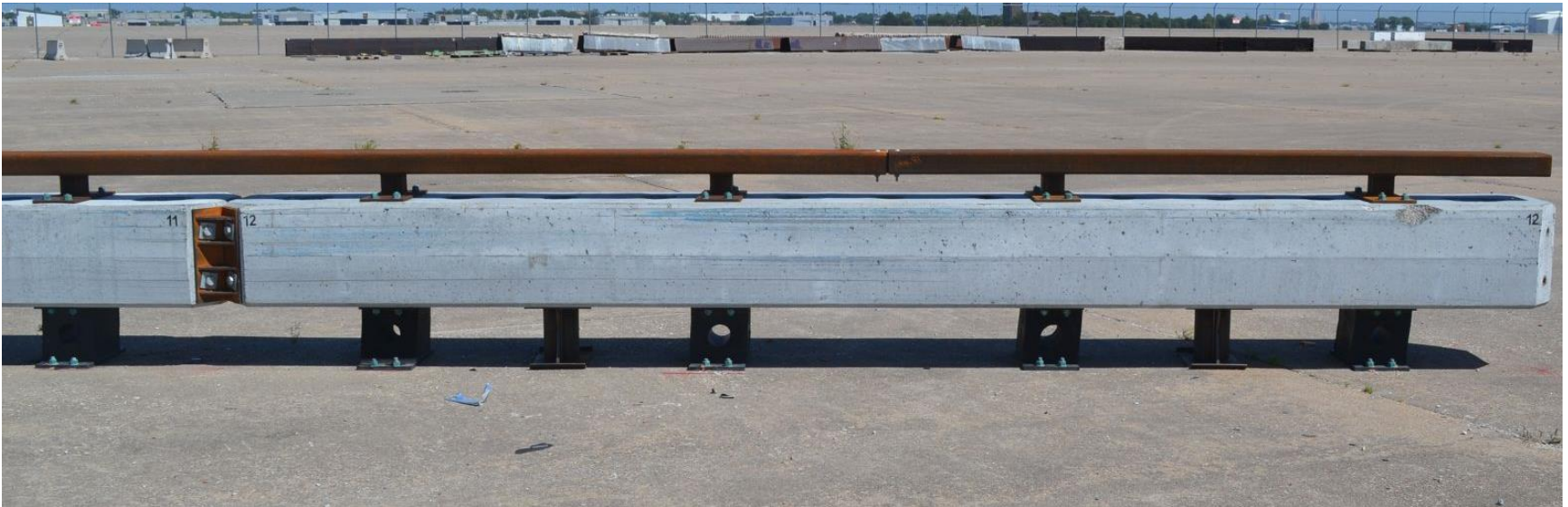
Figure 72. System Damage, Barrier Nos. 11 and 12, Test No. SFH-2
