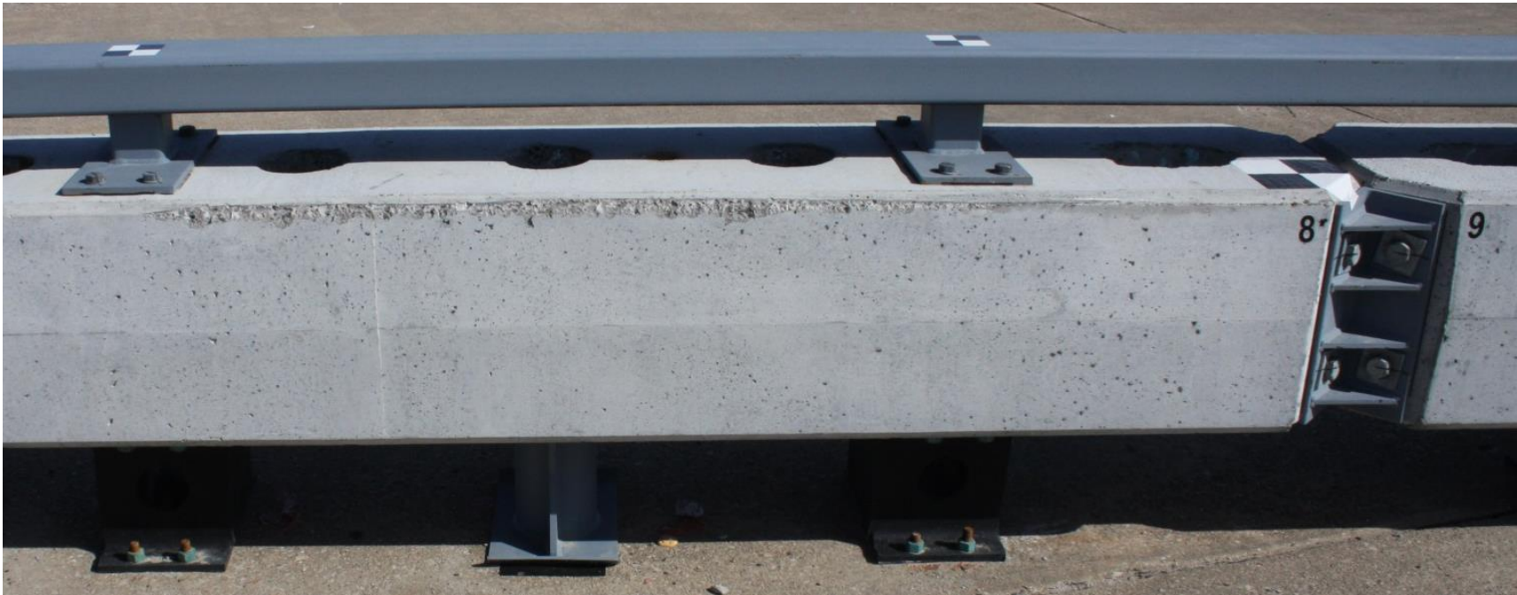
Figure 117. System Damage, Barrier No. 8, Test No. SFH-3
