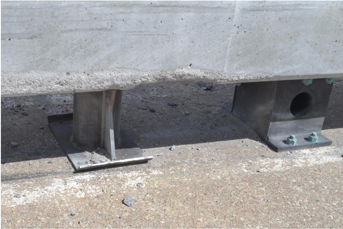
First Skid and Second Post Downstream from Barrier Nos. 5 and 6 Joint
