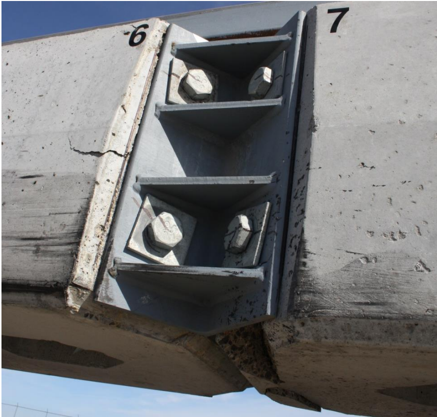
Figure 114. System Damage, Joint between Barrier Nos. 6 and 7, Test No. SFH-3
