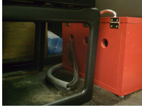
Figure 21. Conduit fed into data collection box.
