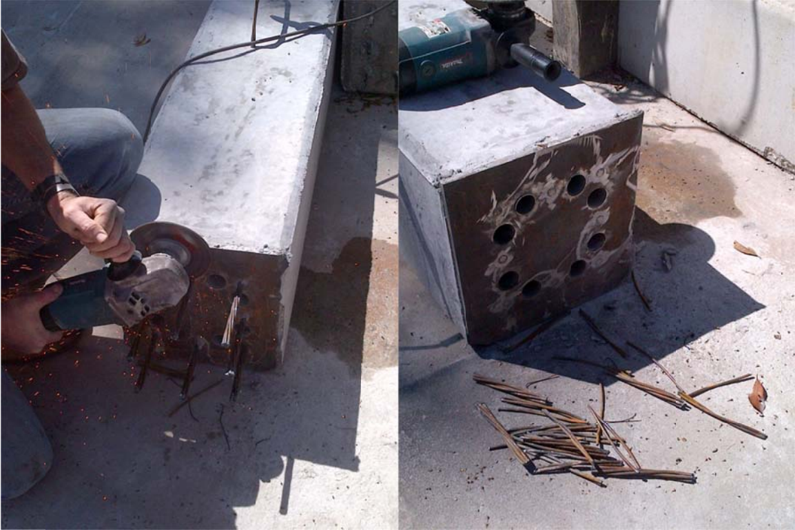
Figure 4.42. Strands cut from jacking (upper) end of upper pile segment.
