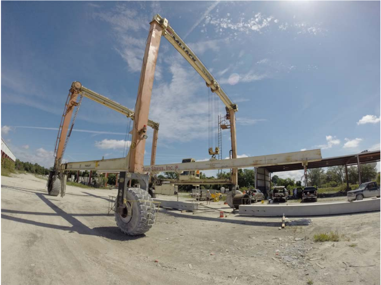
Figure 6.20. Gantry crane used to lift upper pile segment (left) and bring into close proximity with lower pile segment (right).
