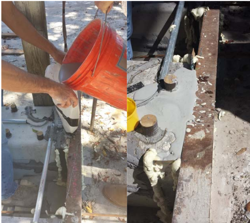
Figure 4.17. Rockite capping compound used to provide intimate contact between piles and header plates.
