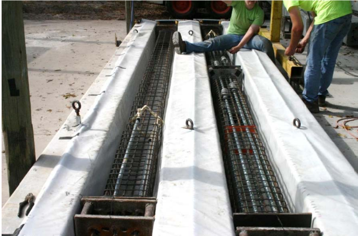
Figure 4.75. Fully stressed bed with spiral reinforcement in place; control pile left, splice specimen right.
