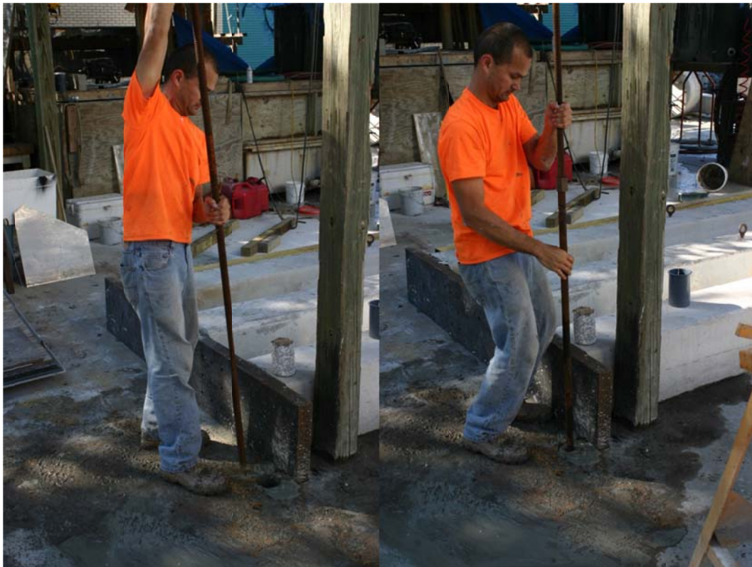
Figure 4.15. Placement of 1in high strength threaded bar, 9ft into grout filled hole.
