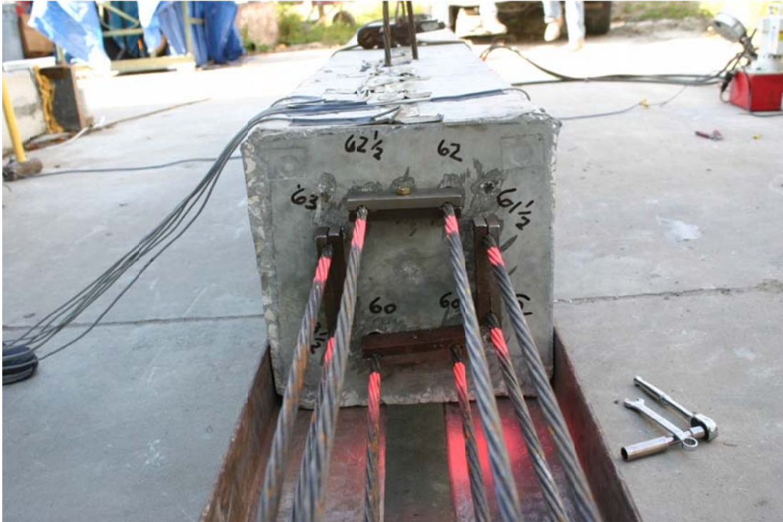
Figure 4.49. All strands in upper pile segment and clamped to prevent inward slippage. Paint stripes show 1.5 in unpainted region to detect whether strands move inward instead of being locked and to show movement was only into lower segment during splice assembly.
