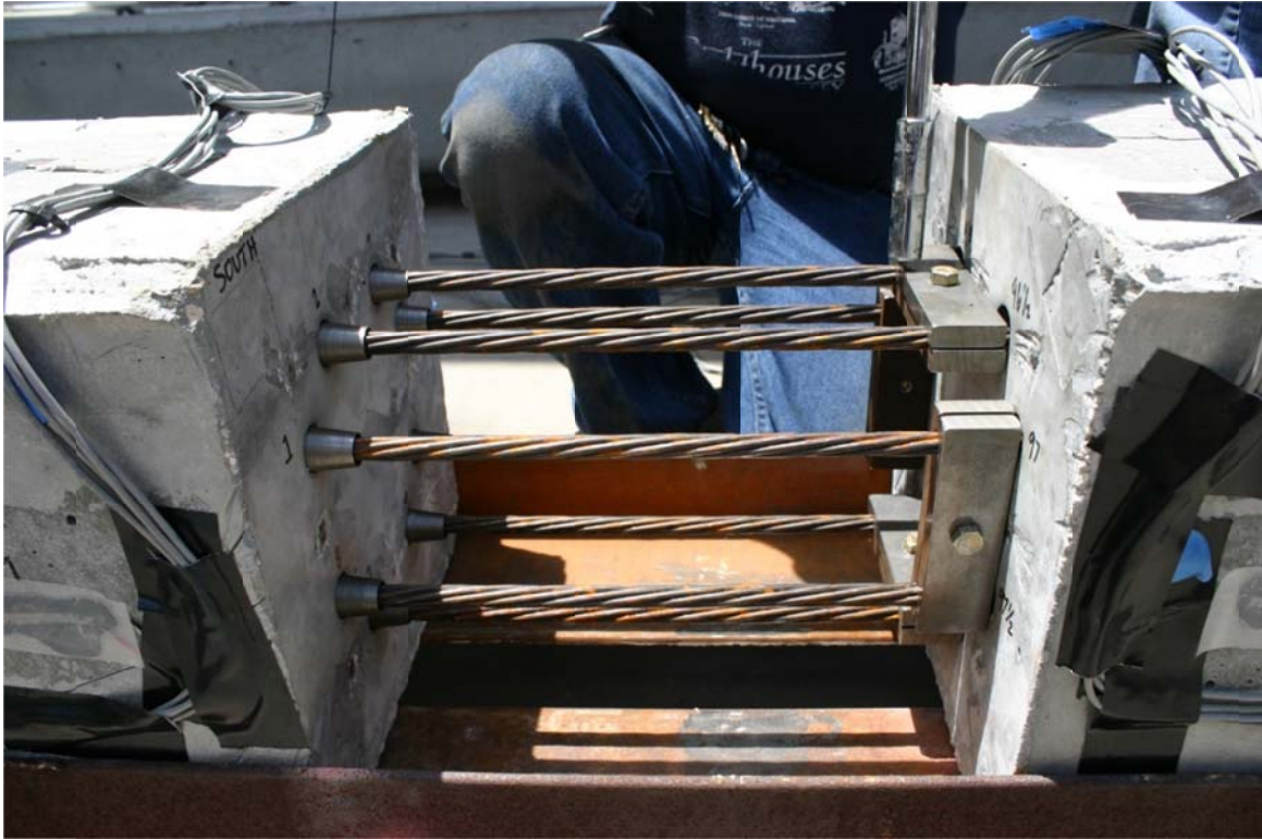
Figure 4.99. All strands embedded past anchorage wedges (lower pile left).
