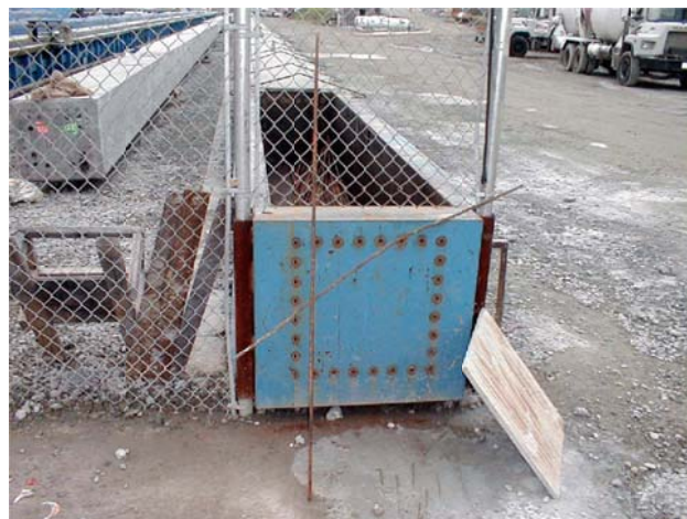
Figure 1.2. Self-stressing, temporary casting beds used for the Haughton Road Bridge in North Carolina to cast solid 30in square piles.
