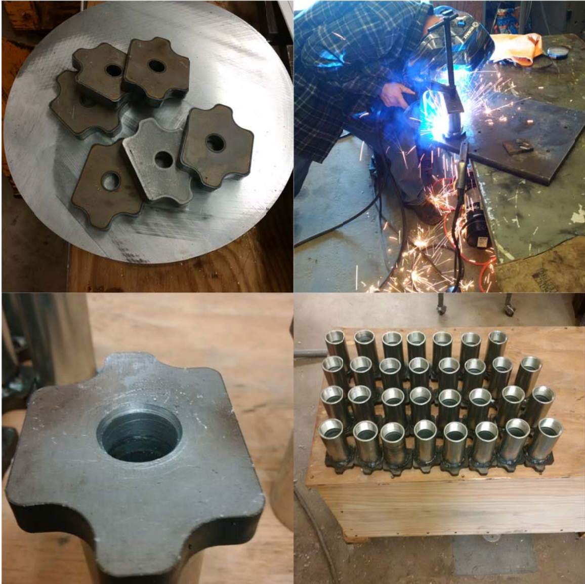
Figure 6.1. Laser cut plates (top left), welding chuck/plate anchorage assembly (top right), machined close tolerance anchorage (bottom left), chucks ready for duct connections (bottom right).
