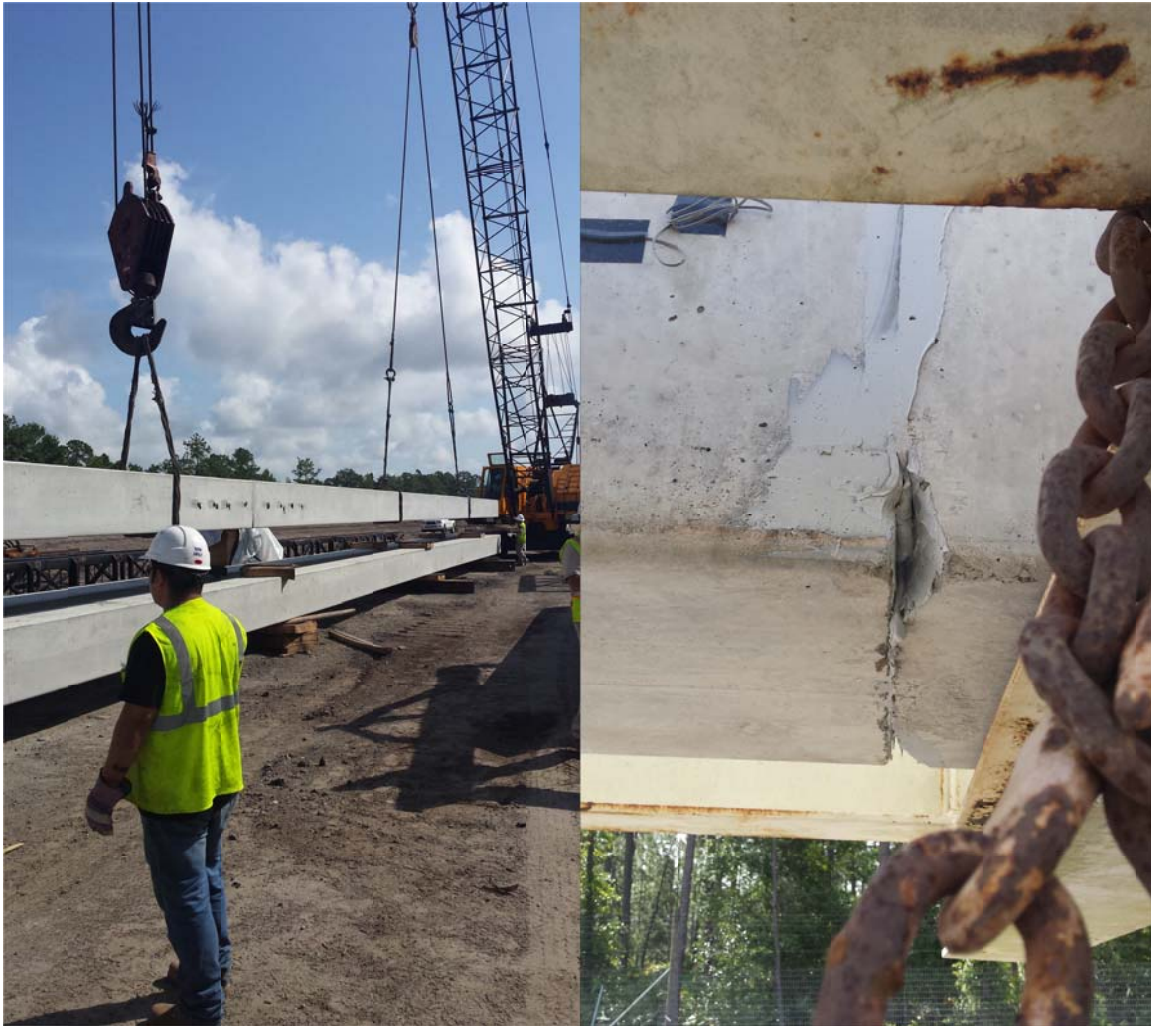
Figure 6.35. Splice pile specimen delivered on-site (left); damaged corners (right).
