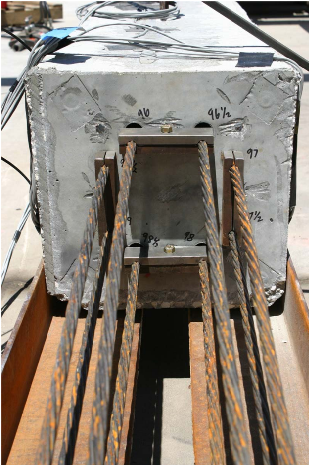
Figure 4.91. All strands in upper pile segment and clamped to prevent inward slippage.
