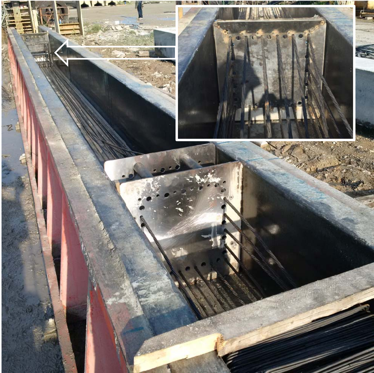
Figure 6.8. Strands threaded through header plates in casting bed, splice header foreground; chamfered jacking plate header (background).
