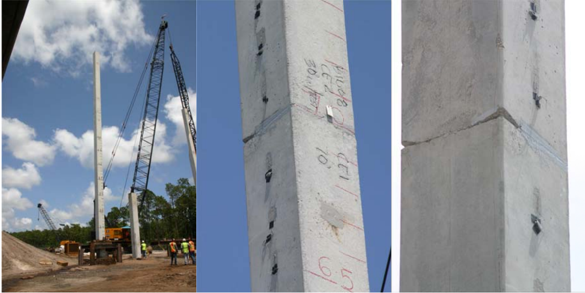
Figure 6.36. Pile in template prior to driving (left); close-up of splice prior to driving (middle and right).
