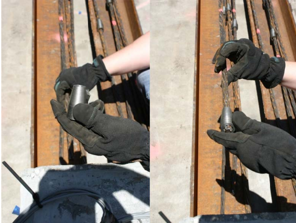
Figure 4.96. Placement of threaded isolation sleeves on strands before insertion into south ducts. Sleeves are designed to prevent epoxy from filling grouting ducts during final contact.
