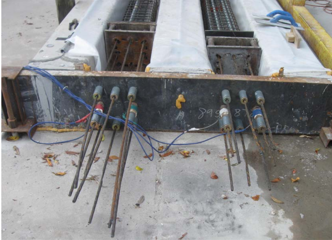
Figure 4.72. Strands in place and load cells on center two strands of each pile on dead end; control pile left and splice pile right.
