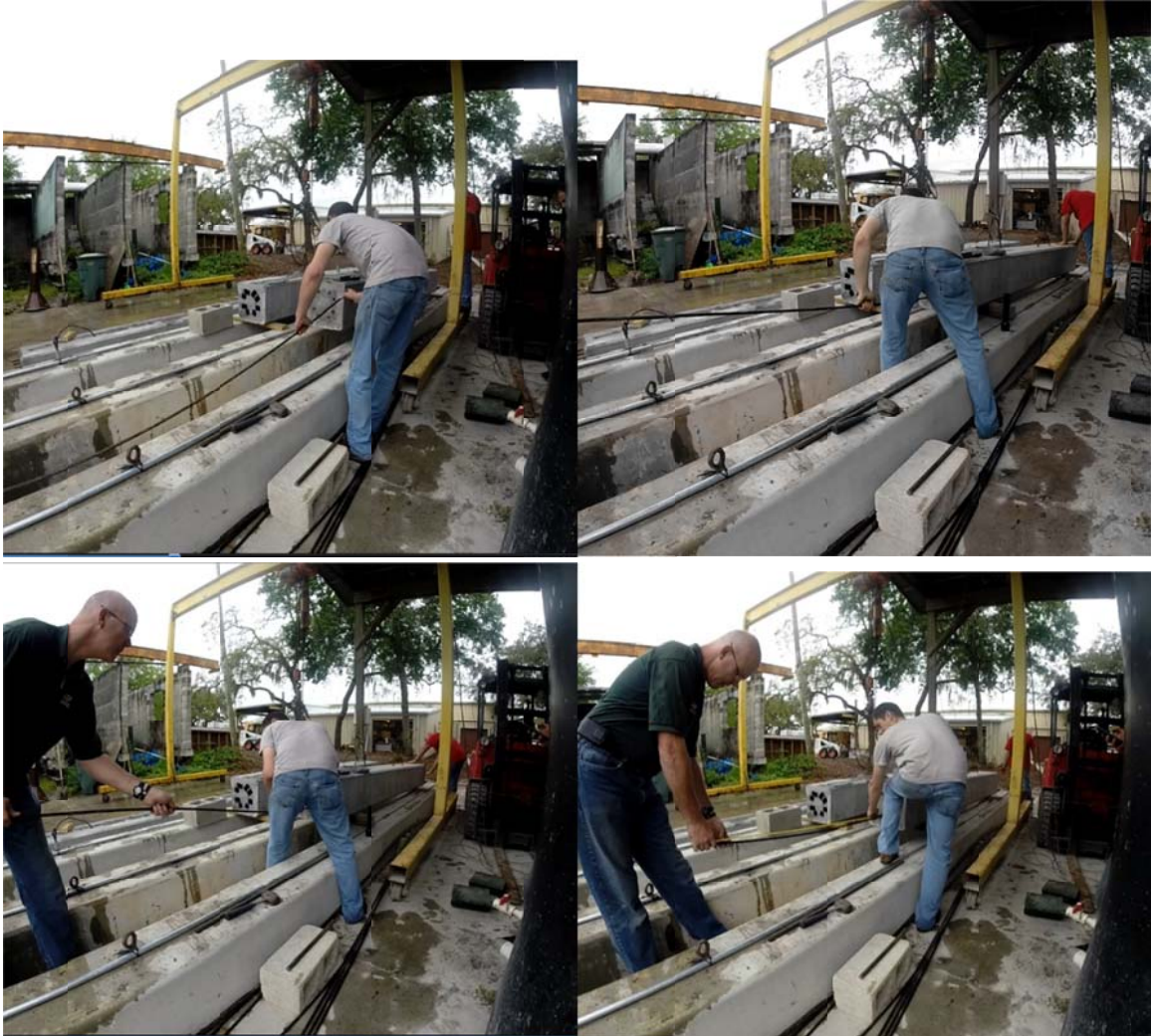
Figure 4.48. Threading strands into upper pile segment. Each strand measured to be \frac{1}{2} in longer than the previous (shortest strand stubbed out 60 in; longest 63.5 in).
