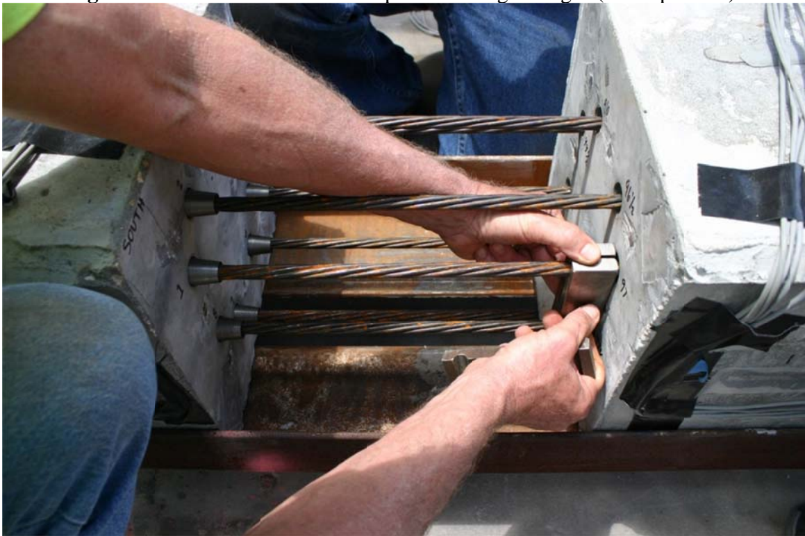
Figure 4.100. With all strands in, strand clamps need to be removed (upper segment right).
