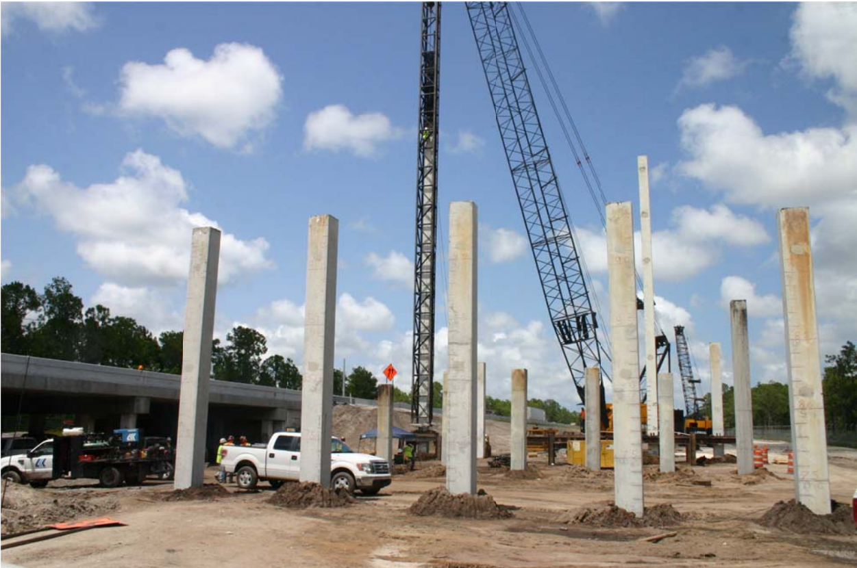
Figure 6.37. Deer Bridge piles looking northeast (End Bent 3-1 in foreground, End Bent 3-3 in background, splice pile in leads driven to the left / northwest of Pile 1, EB 3-3).
