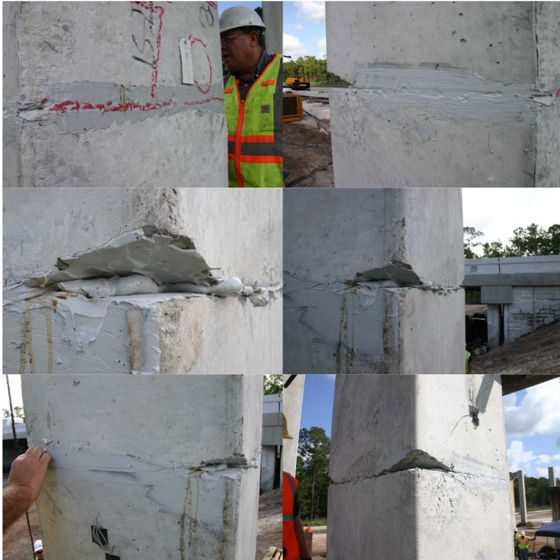
Figure 6.40. Visual inspection of all sides of the pile showed hairline crack in epoxy.
