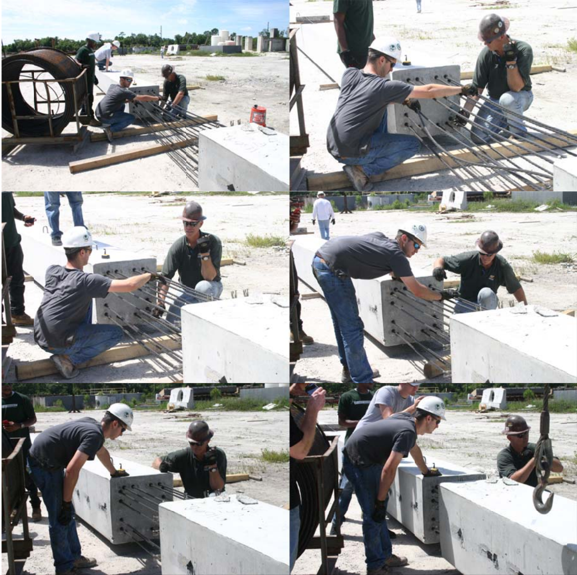
Figure 6.21. Feeding splicing strands into lower pile (background) as upper pile (foreground) was brought closer.
