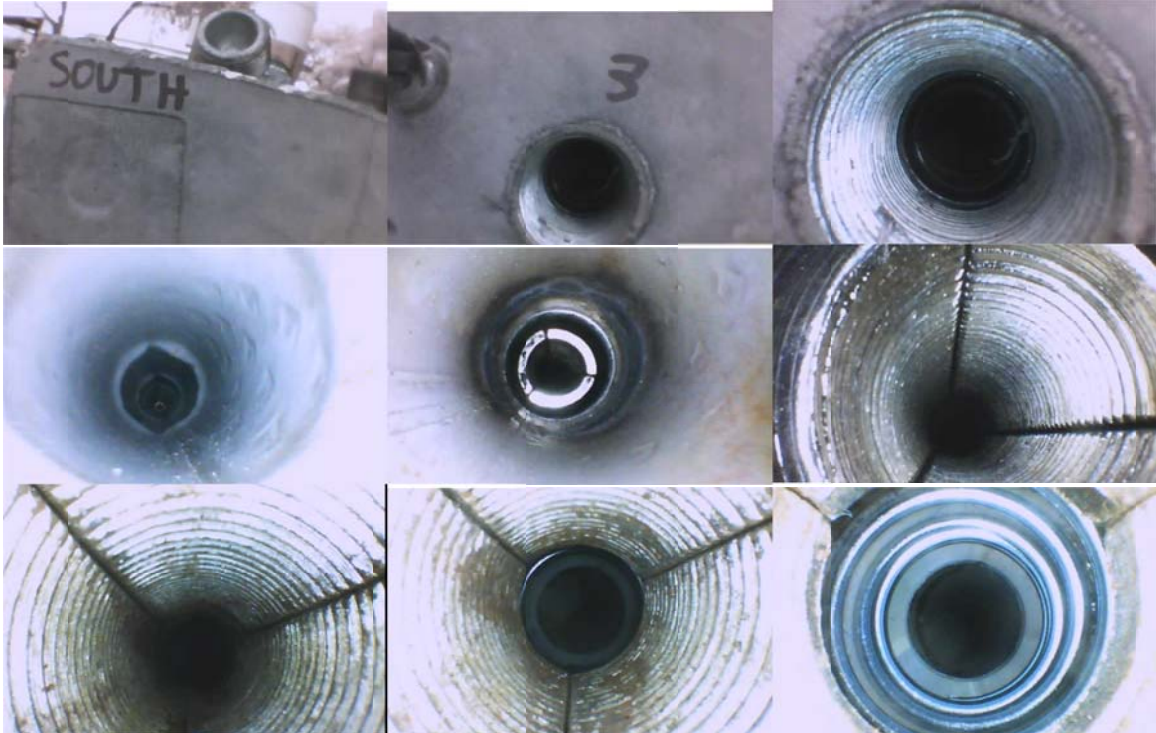
Figure 4.89. Borescope images of duct 3 showing marked reduction in debris near wedges compared to the first splice pile. This reduction in debris is due to the use of threaded duct caps which do not pass through splice header assembly thus eliminating the need to grinding / cutting off the ducts. All ducts were blown out and all debris was removed.
