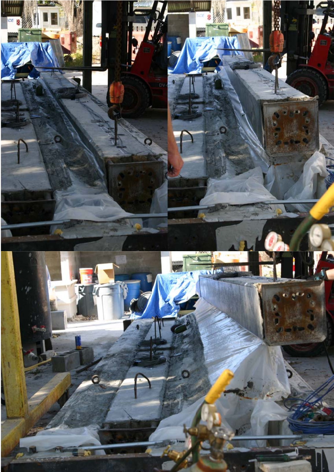
Figure 4.39. Un-spliced control pile extracted from casting bed; plastic bed lining peeled off.
