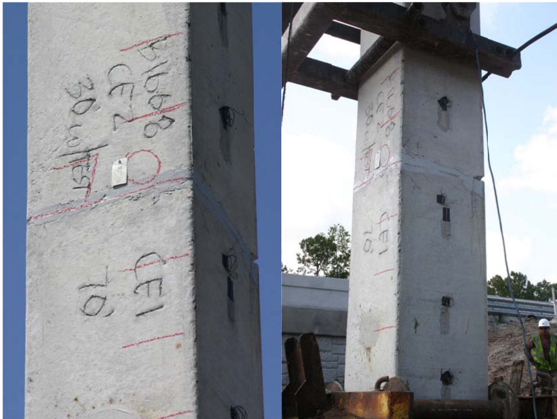
Figure 6.39. Visual inspection of splice at each cushion change (added 7.5in at 44ft, left; replaced with 9in at 76ft, right).
