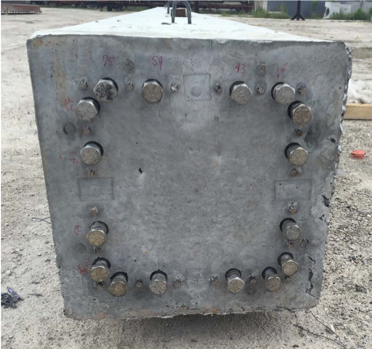
Figure 6.15. Lower pile segment splicing face showing some honeycombing on right side.
