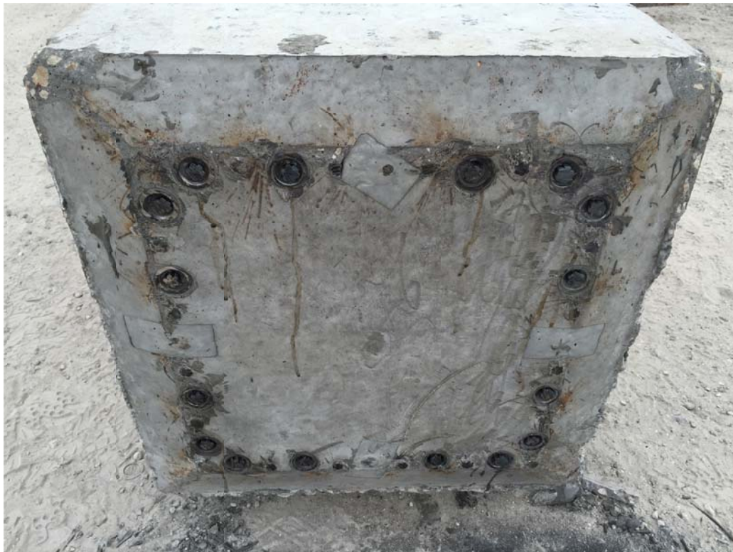
Figure 6.33. Upper pile end with all grout fittings removed and strands cut flush for driving.
