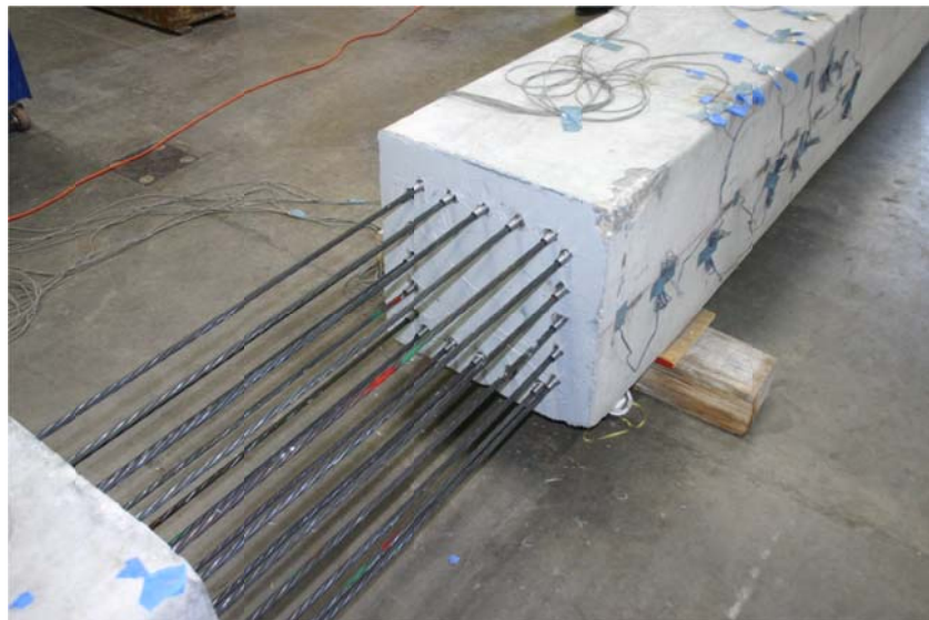
Figure 5.14. All strands inserted passed the lower pile wedges and segments were pushed together.
