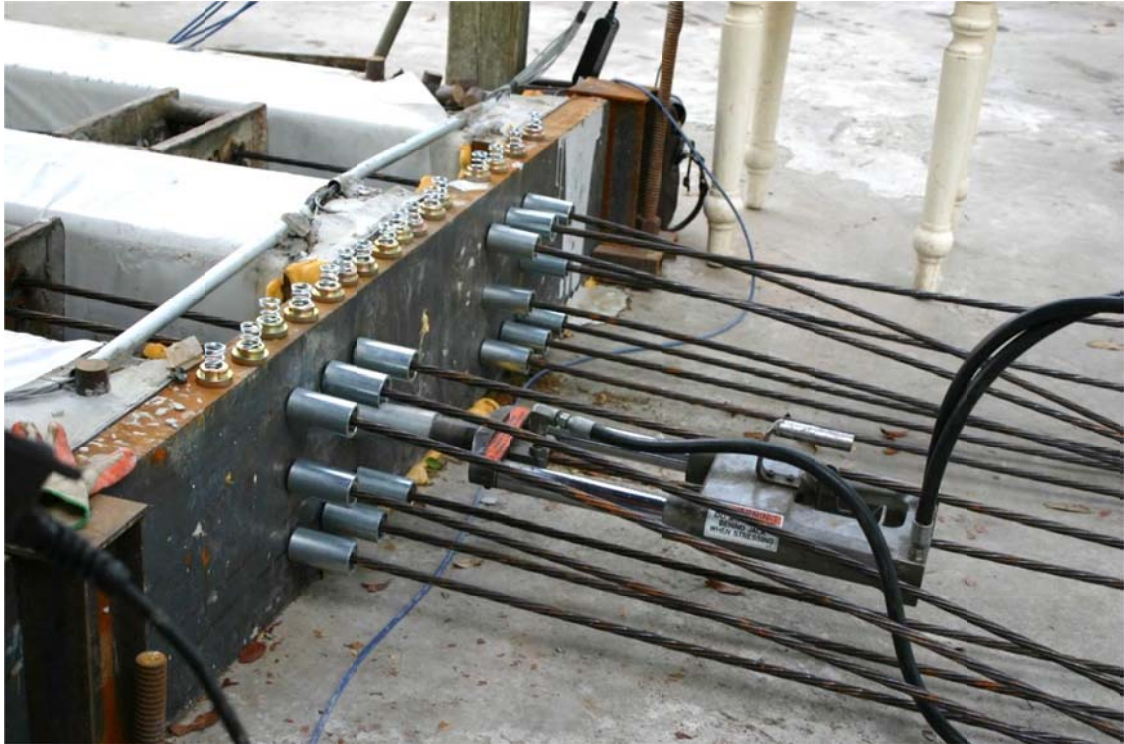
Figure 4.74. Prestressing strands in bed (hydraulic wedge setter used to minimize short bed losses).
