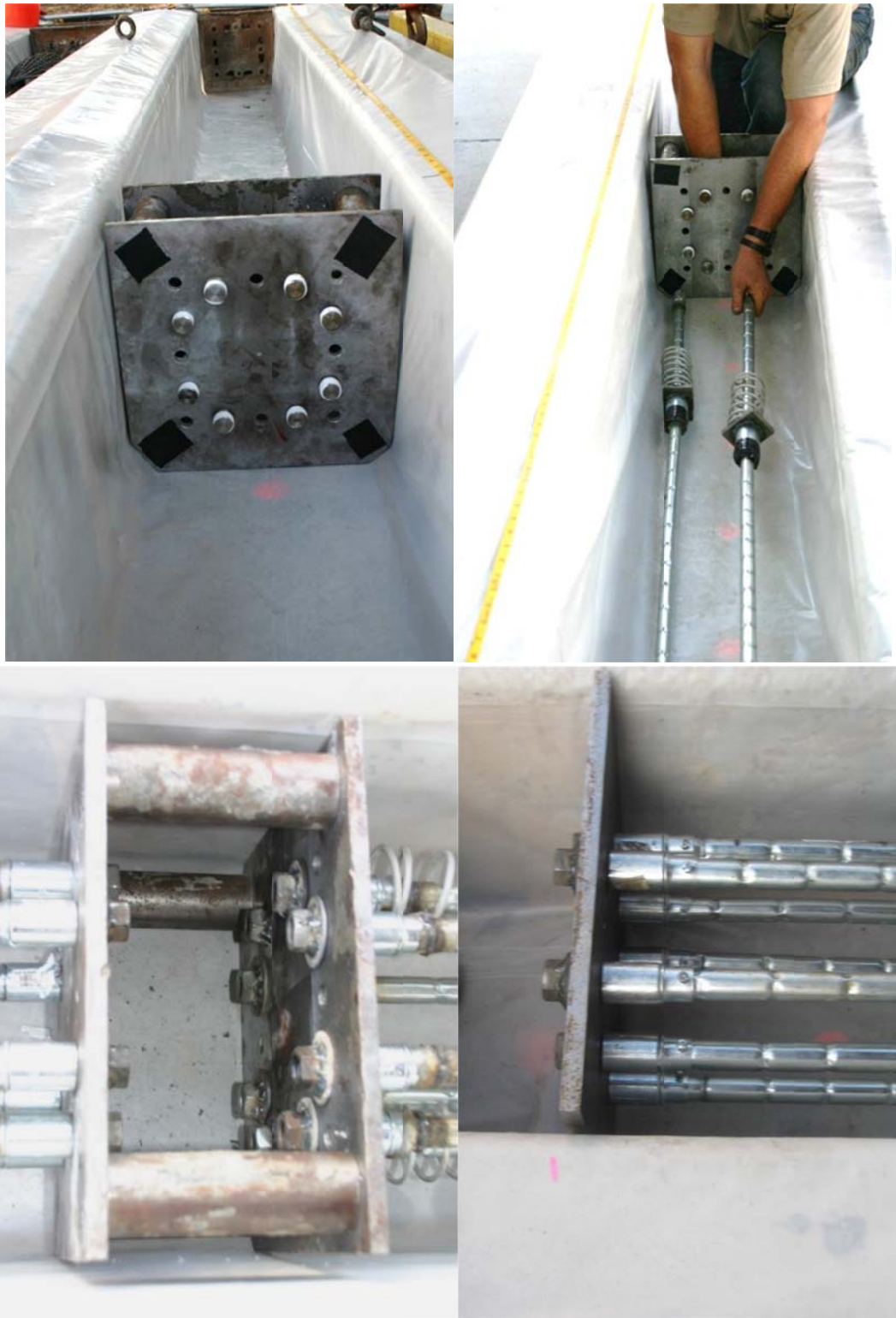
Figure 4.66. Splice header assembly fitted with inserts awaiting installation of ducts (TL); attaching ducts (TR); fully assembled (BR); and jacking end plate at top of upper pile segment (BR).
