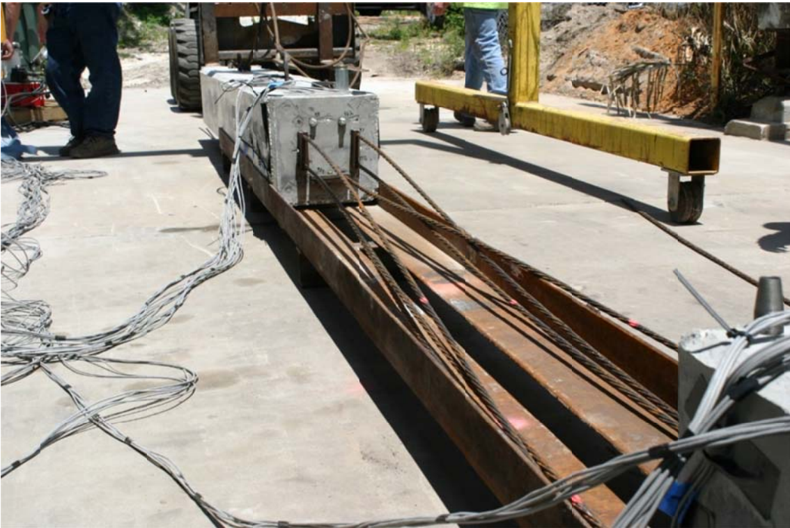
Figure 4.93. Both pile segments on assembly/alignment rail. Upper segment top; lower segment bottom. The paint stripes on strands indicate when each strand will come in contact with the embedded anchorage in bottom pile segment.
