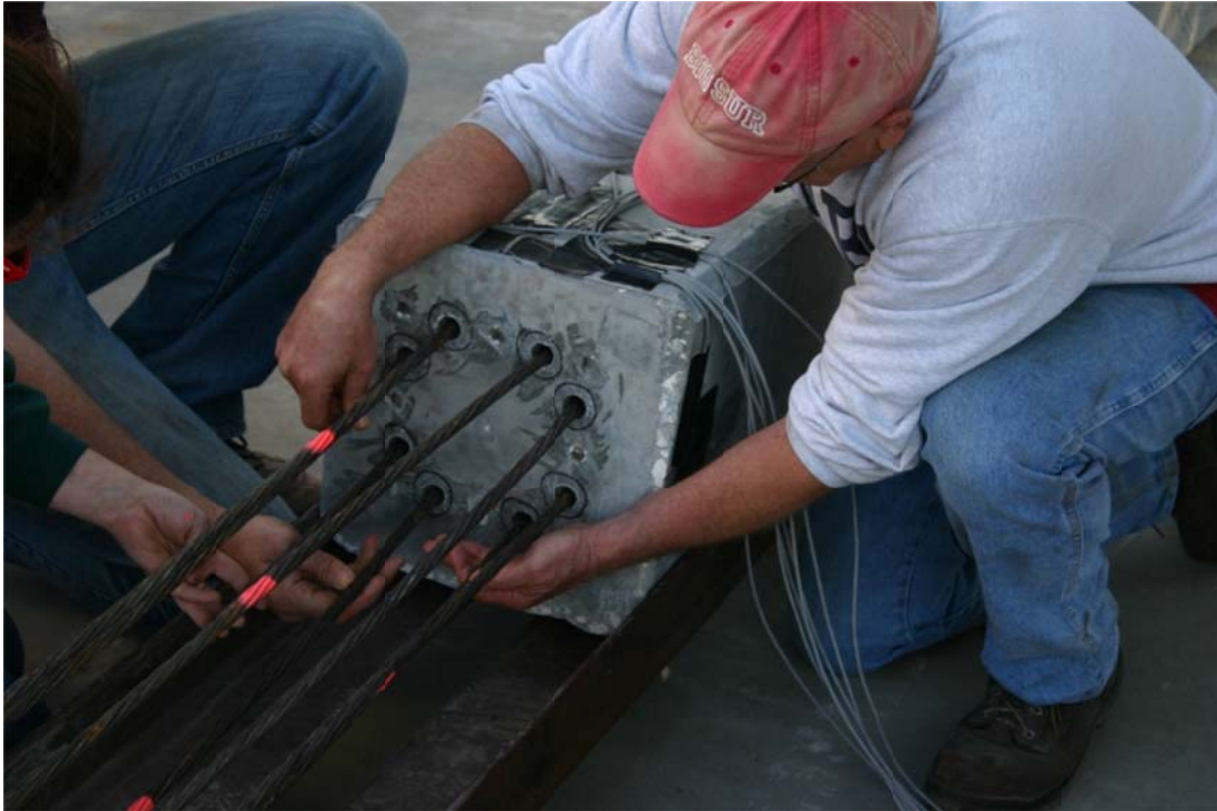
Figure 4.54. All strands inserted. Flexibility of the 5ft strands allows additional options to insert strands at will even if all strands were the same length. However, staggering also meant that no two anchorages were encountered at the same time.
