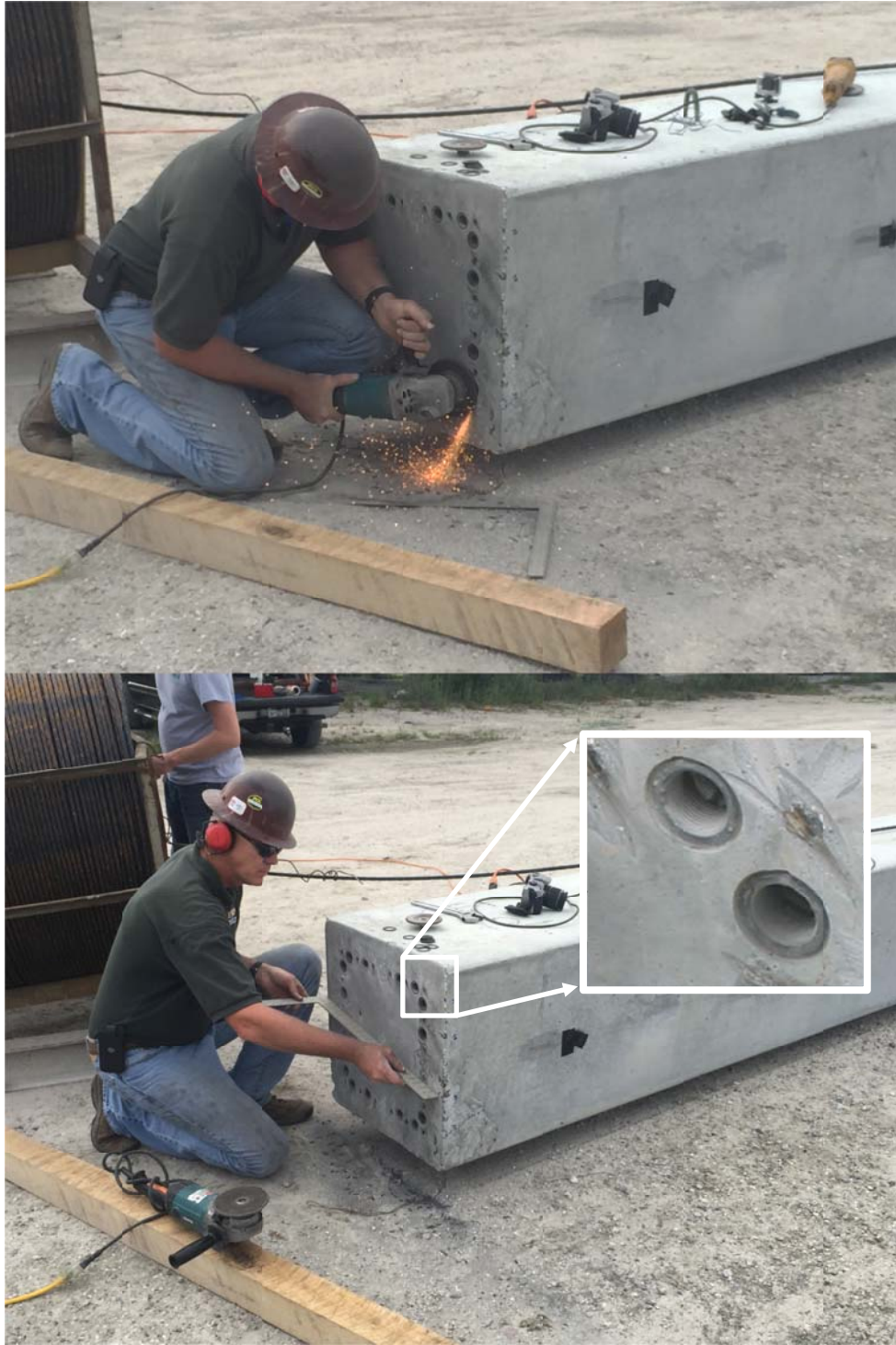
Figure 6.17. Prepping splicing faces by removing high spots from steel strands or concrete edges. Note recessed formed by 1/16in rubber washers.
