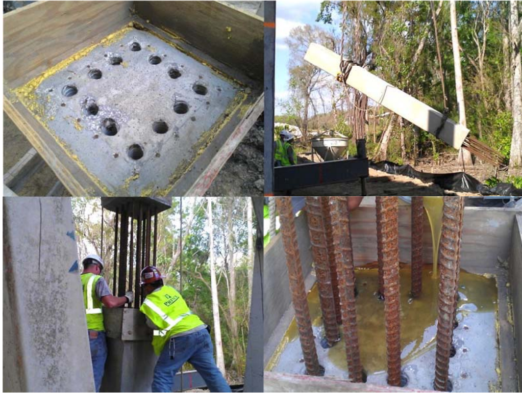
Figure 2.8. Epoxy-doweled splice: bottom pile cored (top left); upper segment cast with rebar hoisted for insertion (top right); aligning rebar while lowering (bottom left); pouring epoxy prior to final descent (bottom right).
