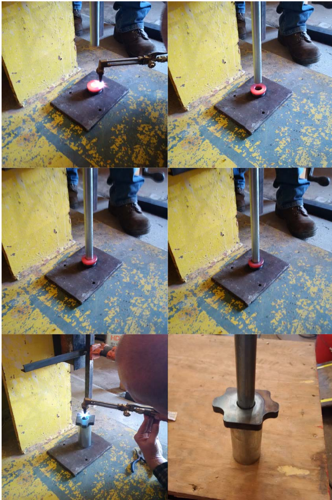
Figure 6.2. Thermal press fitted duct to anchorage process (screw back cap, top four images; bearing plate, bottom).
