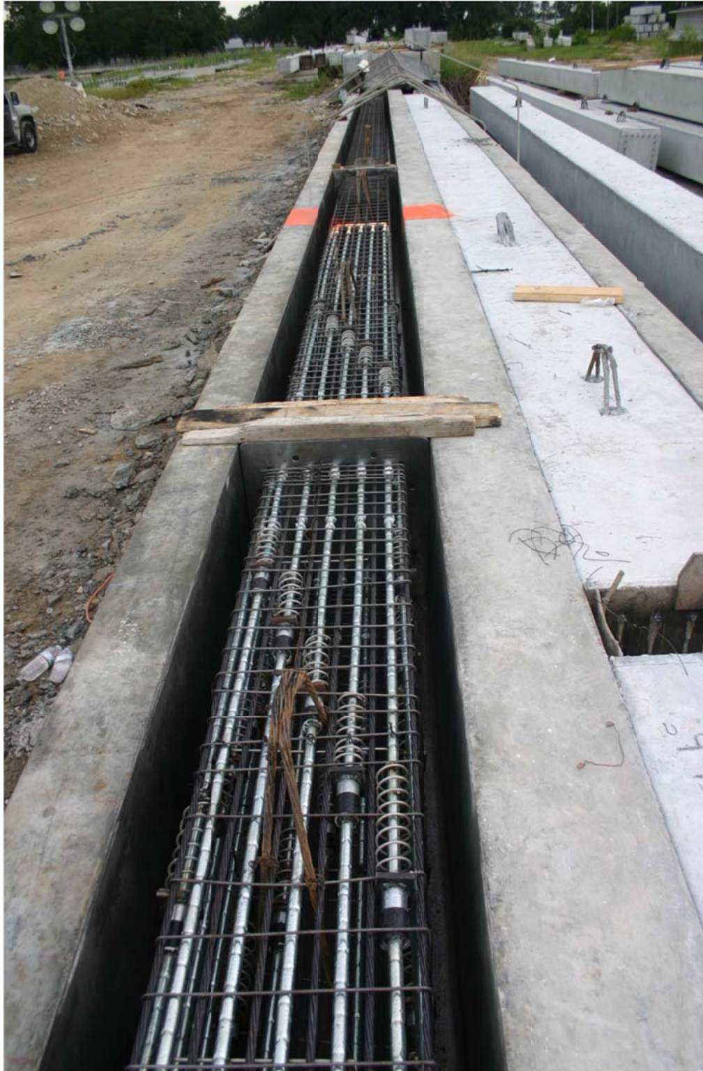
Figure 5.10. Fully stressed bed with lifting loops in-place (note staggered anchorages complete with confinement coils).
