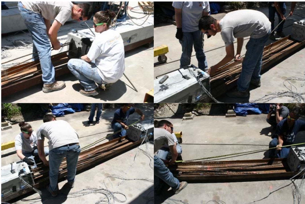
Figure 4.90. Threading strands through upper pile segment. Each strand measured to be \frac{1}{2} in longer than the previous (shortest strand stubbed out 96 in; longest 99.5 in).
