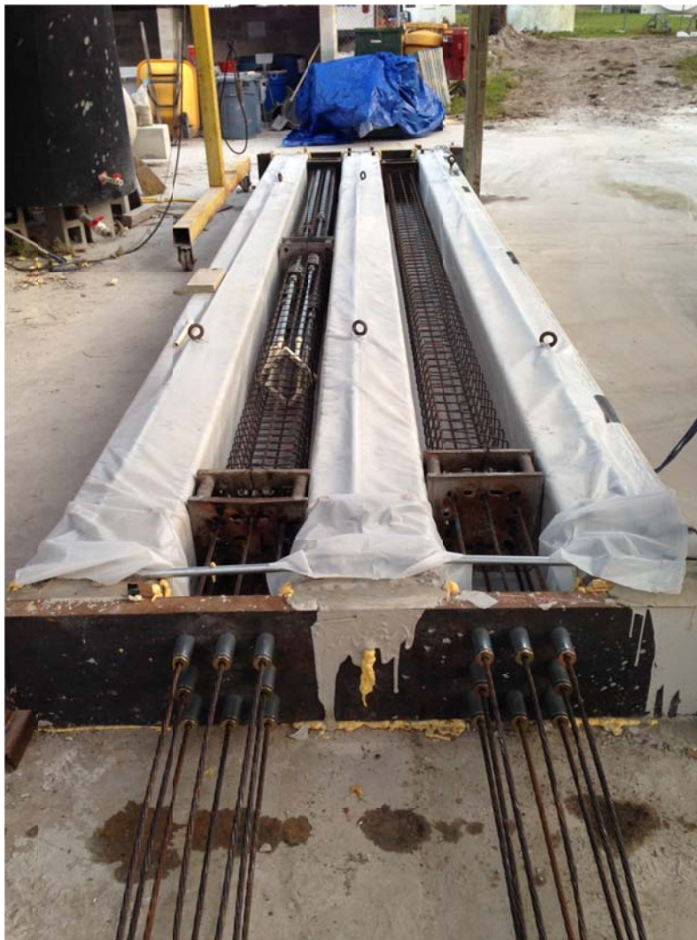
Figure 4.26. Fully stressed bed with spiral reinforcement in place; splice specimen left, control pile right.
