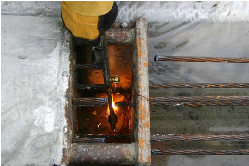
Figure 4.77. Strand cutting after concrete achieved strength; middle splice header (top), and dead end (bot).
