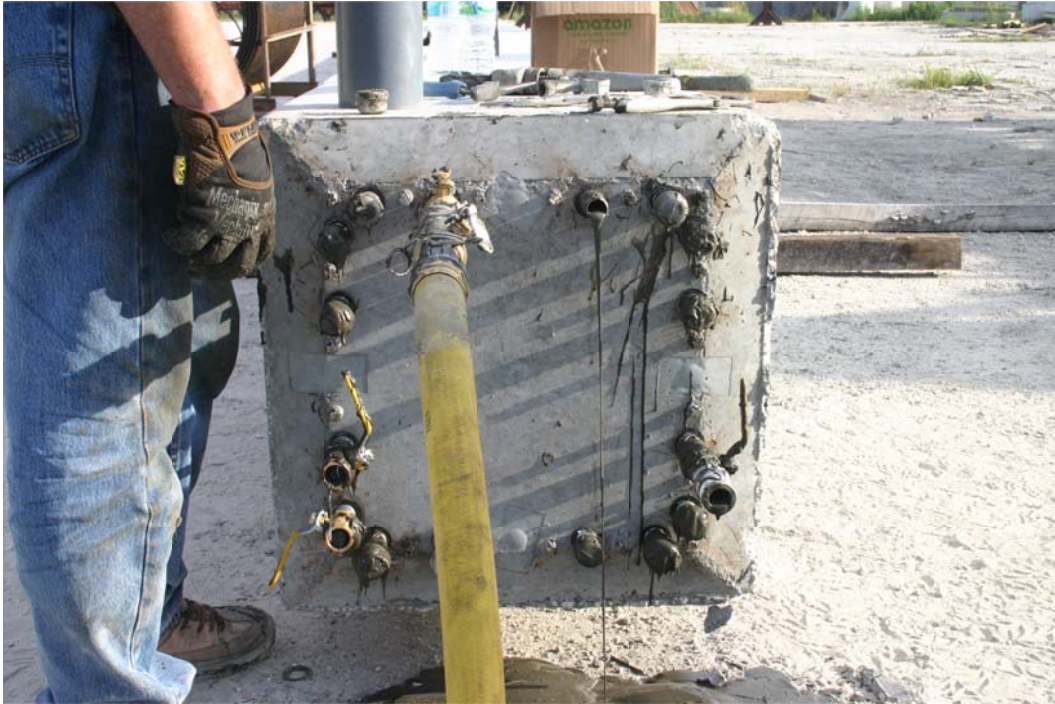
Figure 6.32. Grouting fourth circuit (top) as last duct shows grout return; all others capped.
