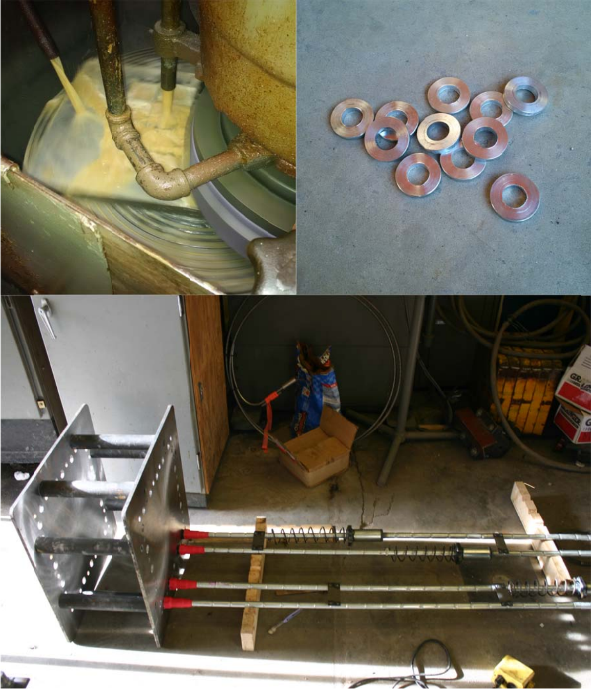
Figure 6.5. Blanchard grinding header plate faces (top left); wedge loss spacers (top right) reconditioned header (bottom) used to pre-fit duct assemblies welded into pairs.
