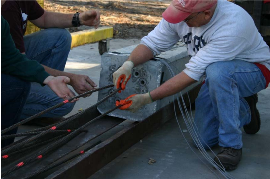
Figure 4.52. Aligning first of 8 strands as pile segments are pushed together. A second paint stripe indicates when each strand will come in contact with the embedded anchorage wedges.
