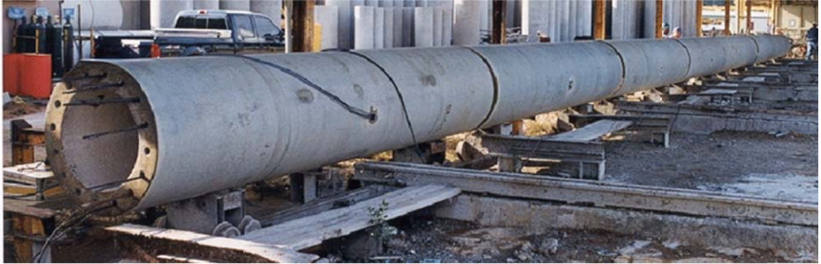
Figure 2.11. Cylinder pile segments aligned with post tension strands in preparation for stressing.
