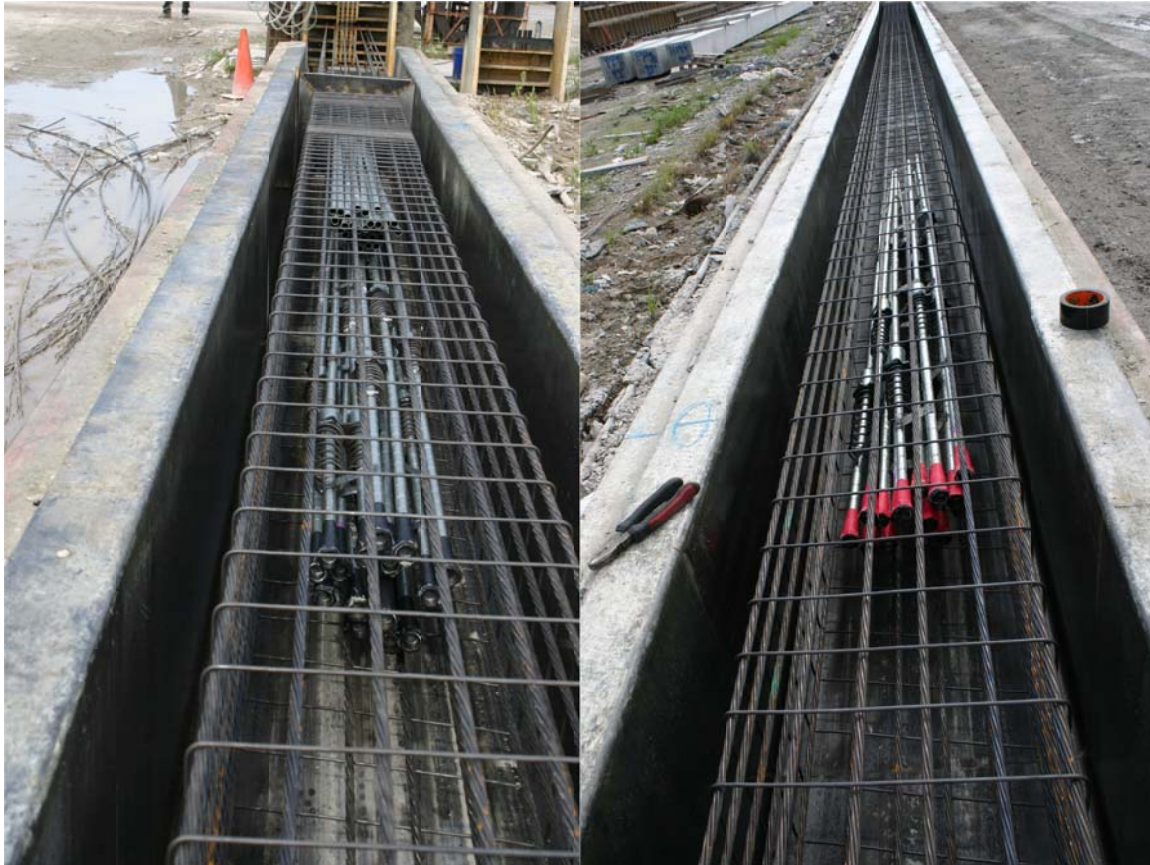
Figure 6.9. Duct extensions and anchorage assemblies suspended with tie wire while spirals were set at prescribed spacings of 1, 3 or 6 inches per standard specifications (upper 30ft pile, left; lower 70ft pile, right).
