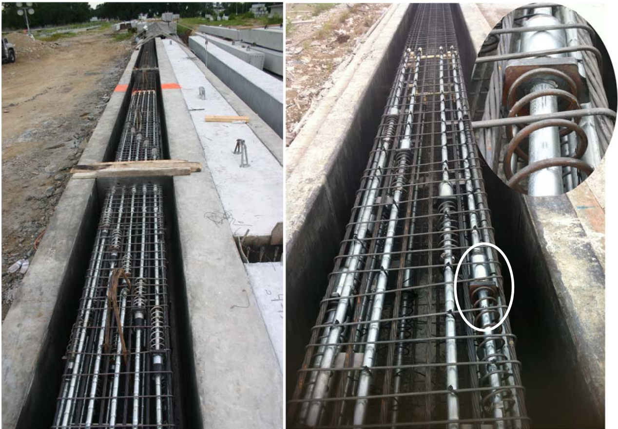
Figure 6.11. Four duct adaptation increased concrete access/flow (right), previously used 5 duct version (left), sculpted bearing plate shape (top right).
