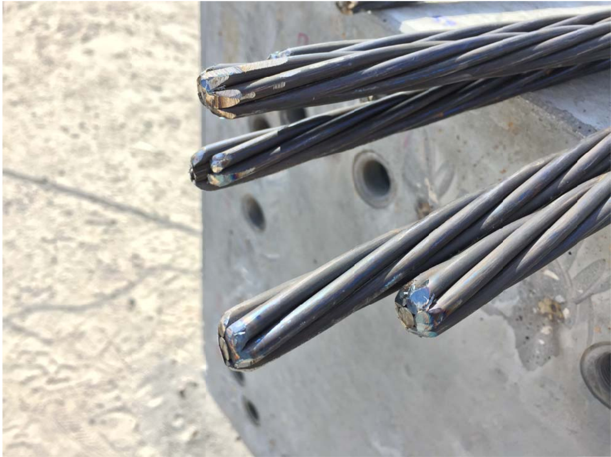
Figure 6.18. Splicing strands ground to removed burrs and sharp edges facilitating easier insertion into embedded anchorages.
