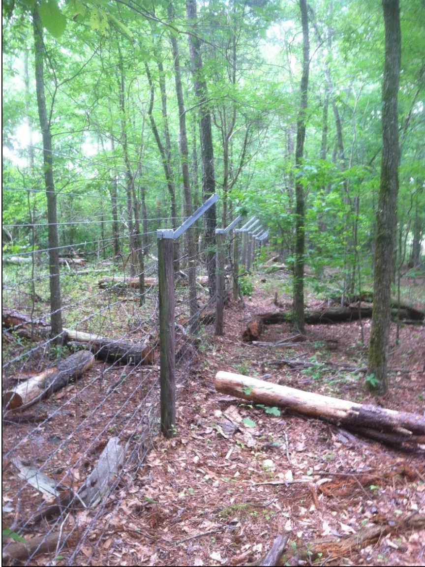
Figure 2. Completed outrigger fence extending from Exit 114 to Bethany Road in Madison, Morgan County, Georgia, USA.
