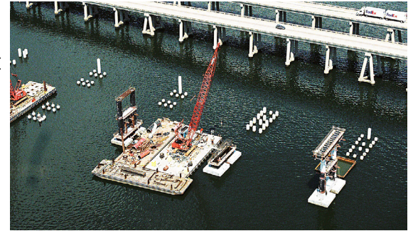
Arrays of piles have been placed, and a barge is used to set the columns which will carry the roadway.
